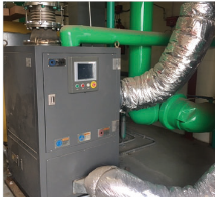
Wastewater Process Equipment
