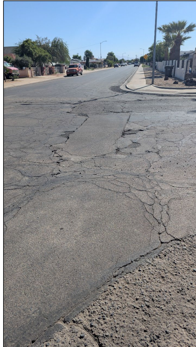
Figure 1 – Roadway deterioration due to improper stormwater retention.
