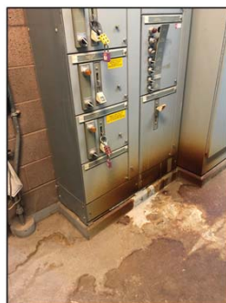
Wildcat Hill WRP Electrical
