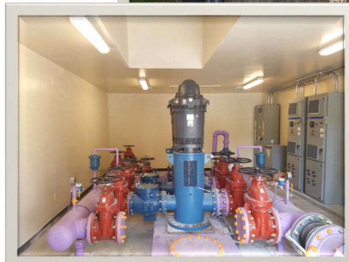
Bushmaster Park Lift Station
