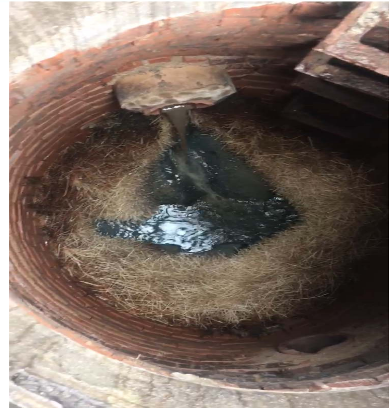
Old brick lined Manhole with root mat at bottom
