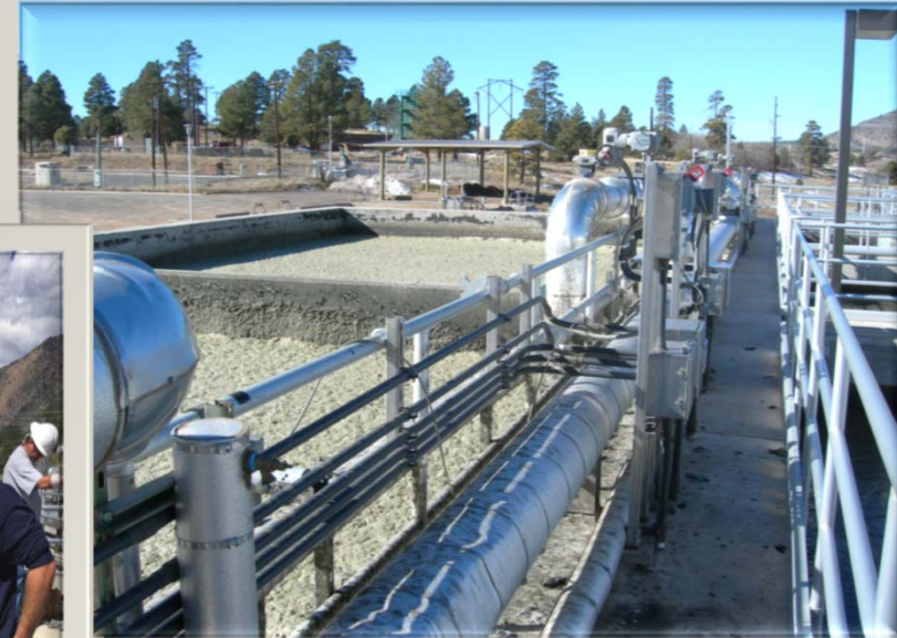
IFAS wastewater treatment basins
