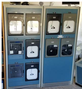
Lake Mary WTP Control Room
