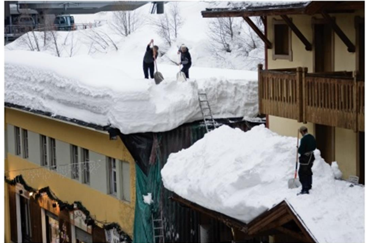
Damage to roof due to large snow loads
