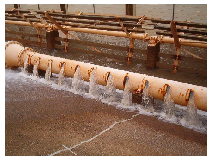
Inlet flow distribution piping corroding
