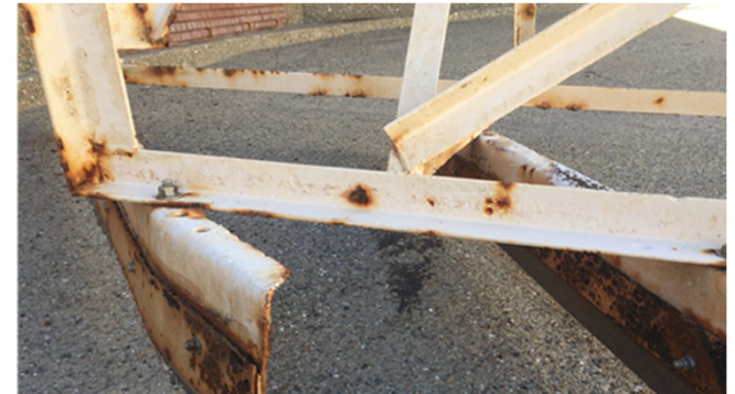
Clarifier Scraper Blades
