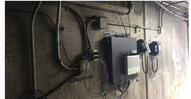
Electrical Wiring in Equipment Tunnel
