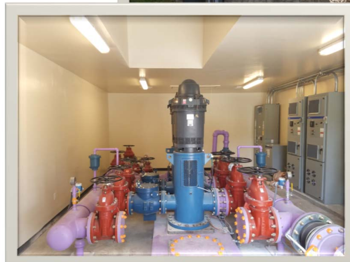
Bushmaster Park Lift Station
