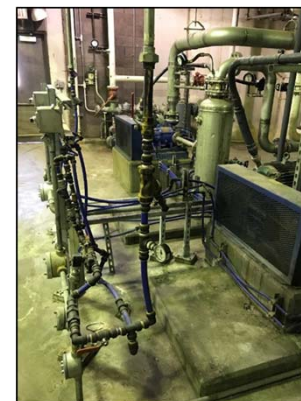
Wildcat Hill WRP Mechanical
