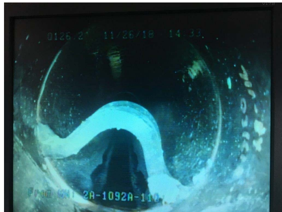
Sewer TV inspection shows gasket installed wrong
