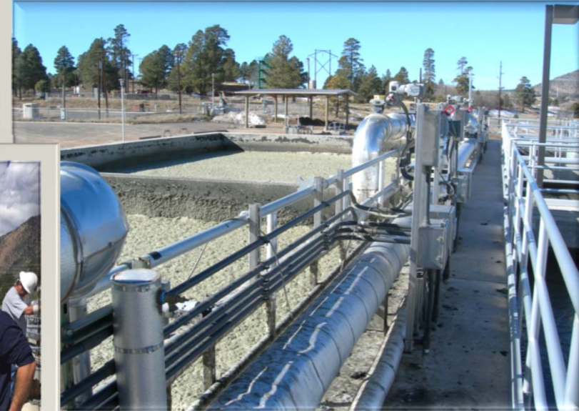
IFAS wastewater treatment basins
