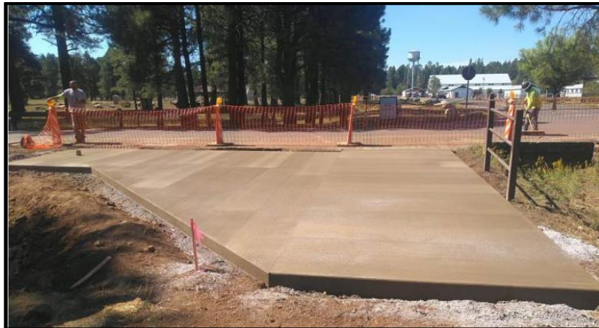
Far western portion of the trail at the intersection with the Sinclair Wash FUTS Trail. This picture shows the color-integrated concrete.
