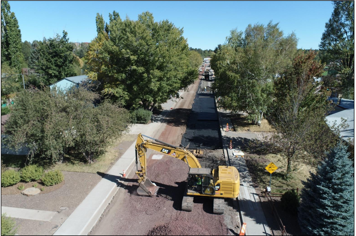
New curb/gutter, sidewalk, and driveways, with roadway demolition and subgrade prep, looking east on Navajo Road
