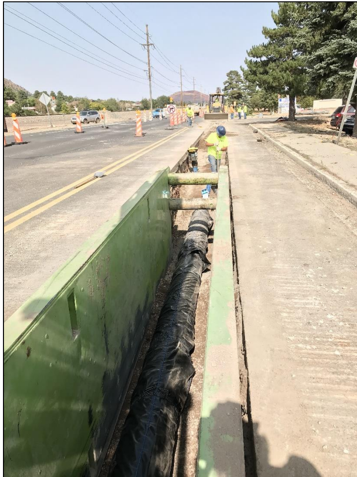
Crews installing last legs of new waterline before the tie ins at the intersection., Industrial Dr., looking East
