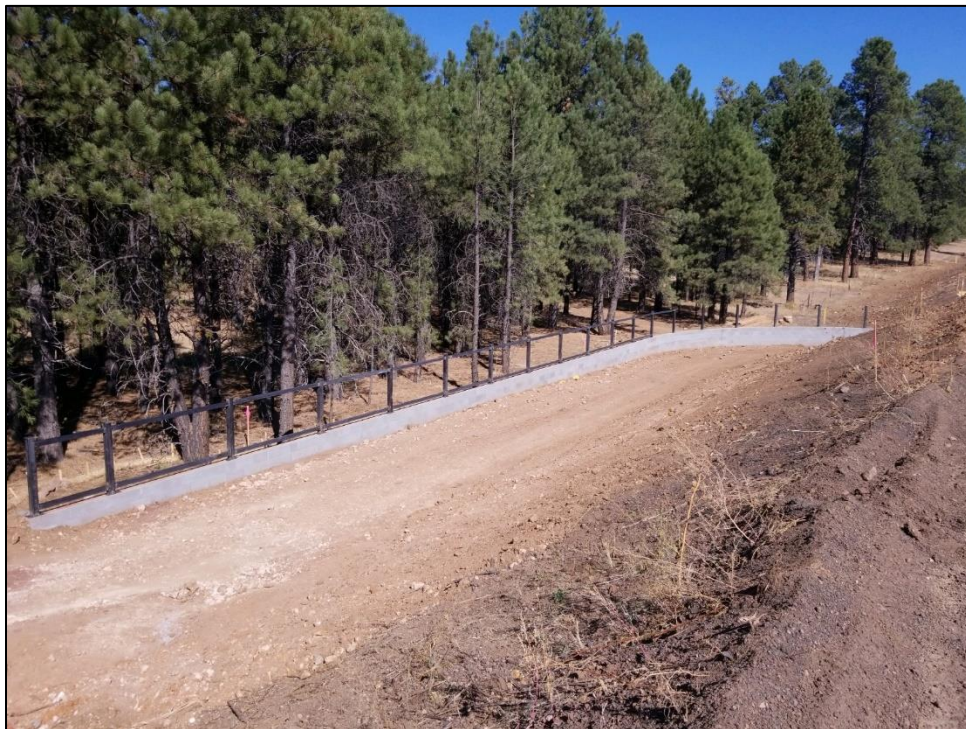
Beginning of the FUTS safety fencing installation on the west side of tunnel
