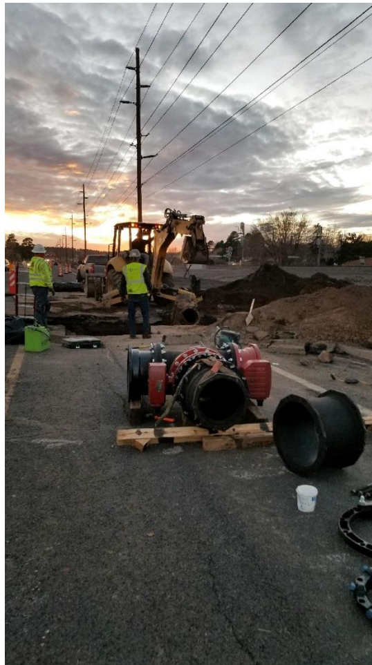
Crews installing last tie in from new watermain to old watermain., Industrial Dr., looking west
