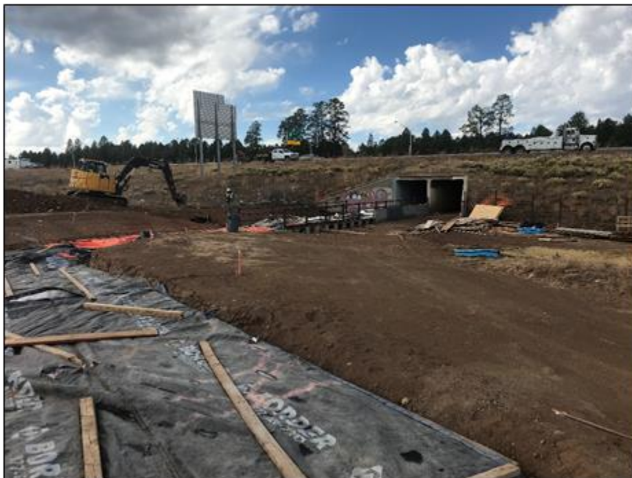
The 10-barrel scupper is complete on the east side and FUTS safety rail is being installed. Tarp/blankets in this picture are to protect the curing concrete from nighttime freezing temperatures.
