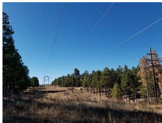
Picture 24 - Powerlines along northern edge of Property from Corner 2 to Corner 1
