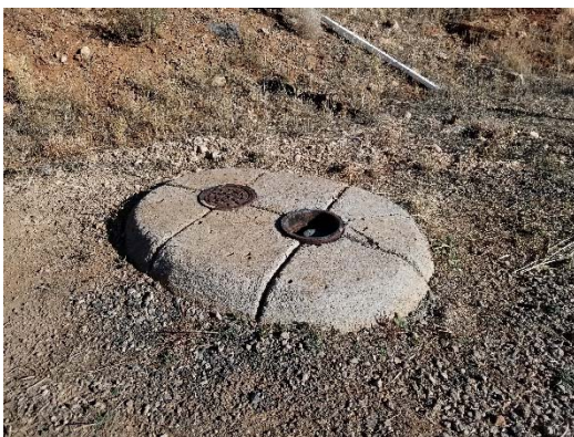
Picture 41 - Water valve located west, outside of west entrance on JW Powell Boulevard
