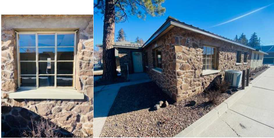
Windows 5 Metal Windows were poorly cut out and Replaced with these fiberglass windows
