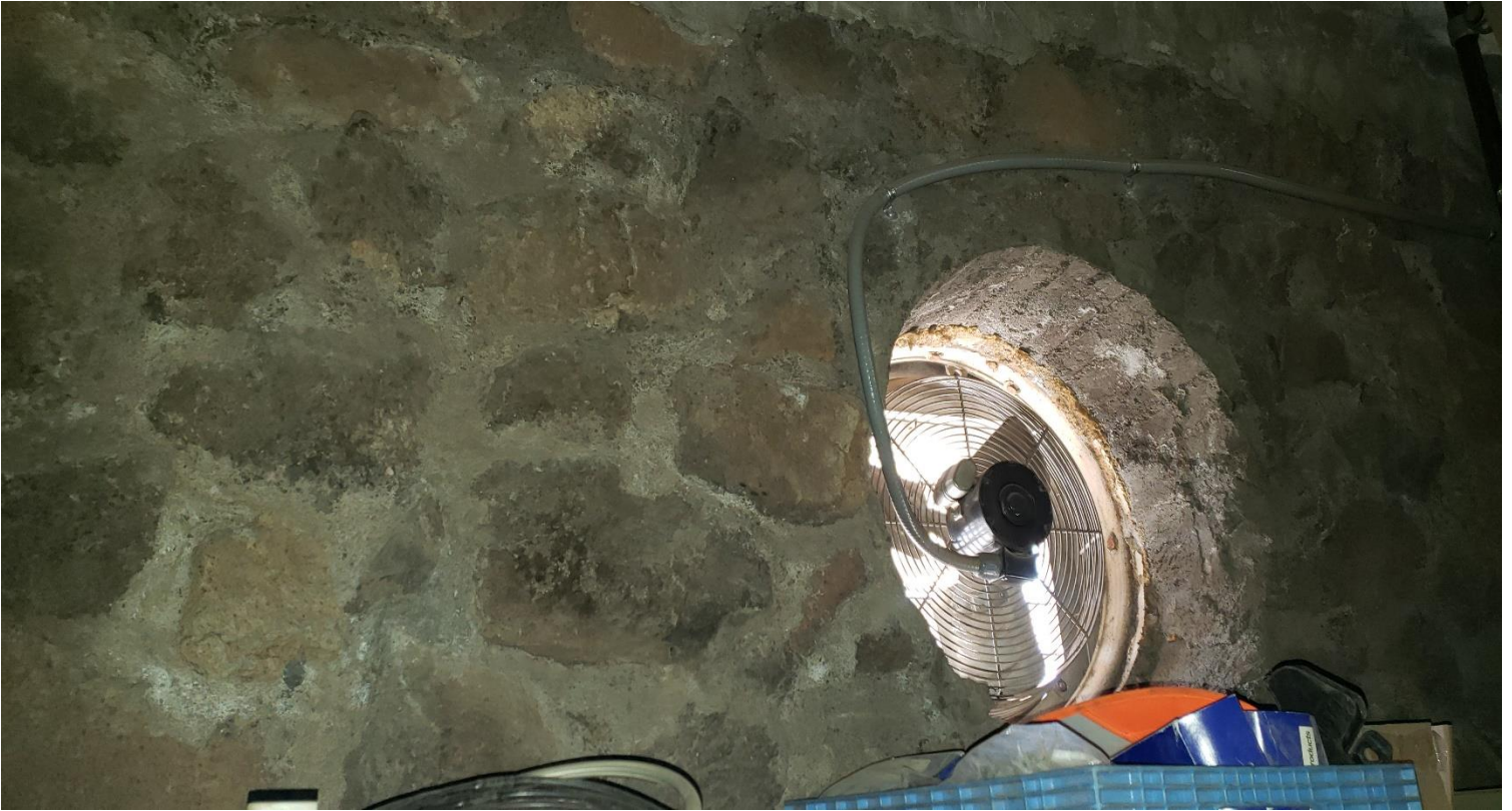
14 S Leroux St interior S façade porthole window, remnant of original garage structure, December 2019.
