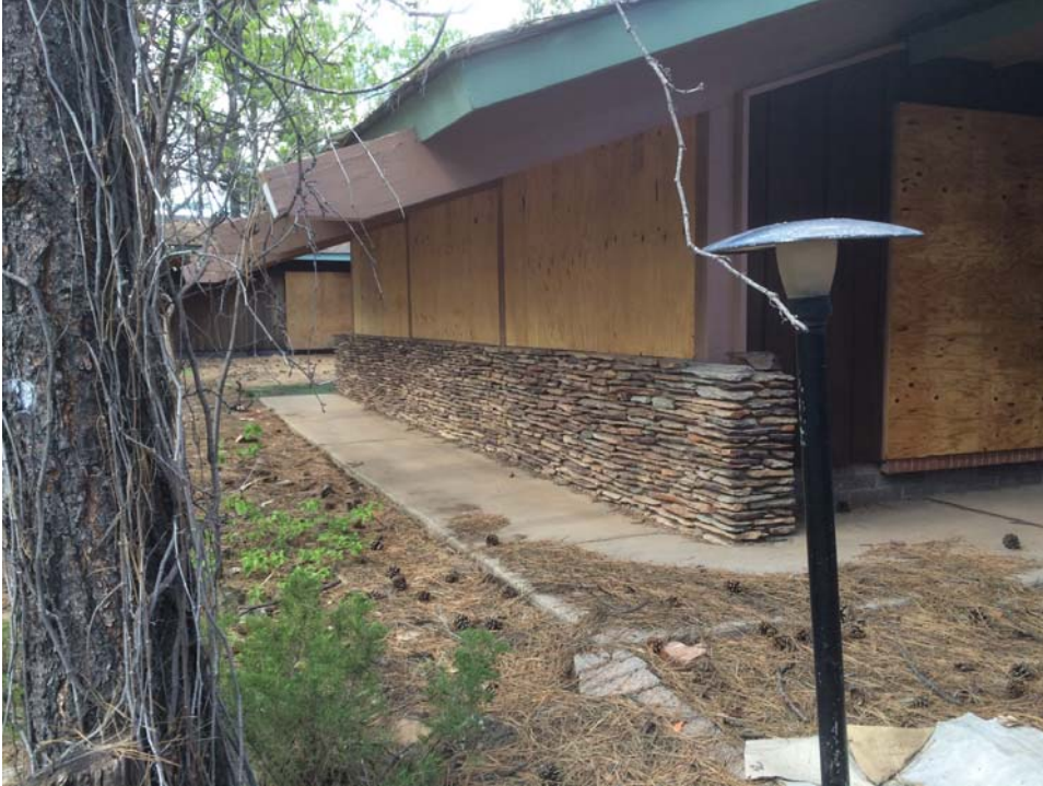
Figure 31. Photograph of the western elevation of the residence, showing the windows and doors of the central living area and north wing covered in plywood.
