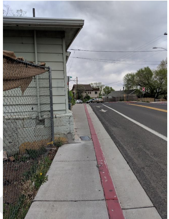
Figure 22: Encroachment into the City right-of-way on Franklin Avenue
