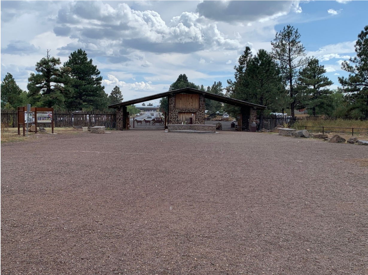
View of the entryway from inside the park. New concrete at the entry will help make it more accessible. Sign kiosk is at left
