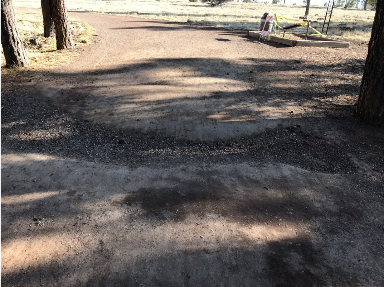
Locations along the trail where water is causing erosion will be fixed via the grant
