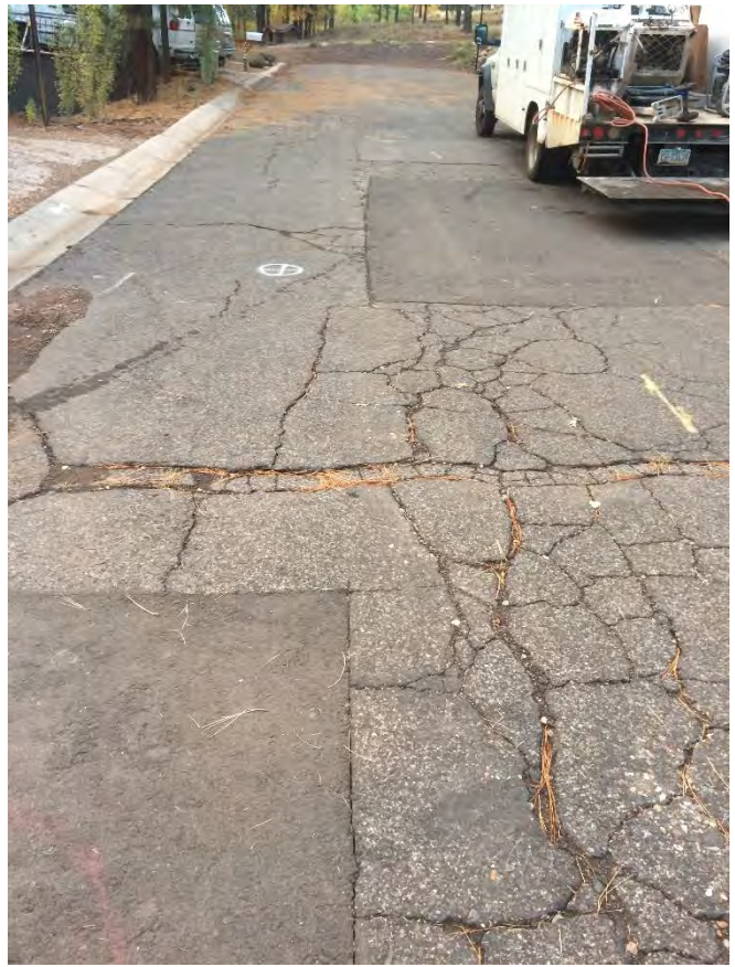
Photo No. 2: Advanced block cracking and utility patches on Canyon Terrace Drive
