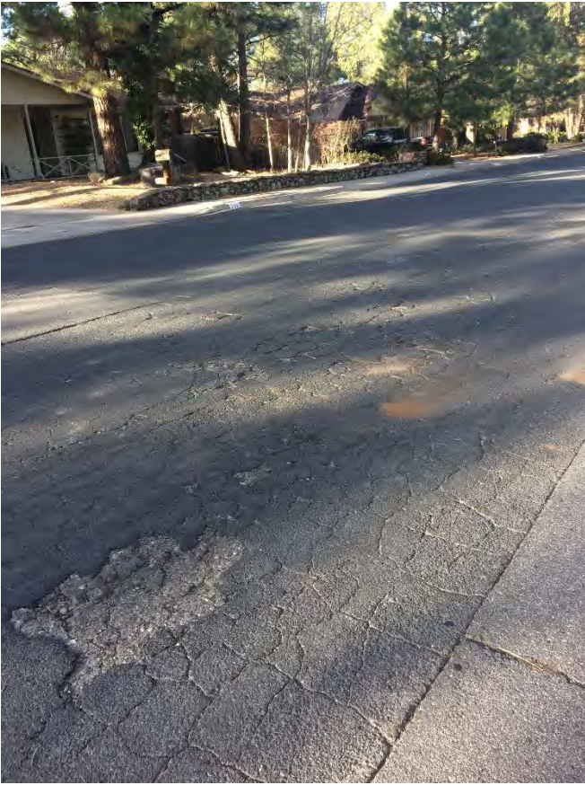
Photo No. 1: Alligator cracking on Hutcheson Drive
