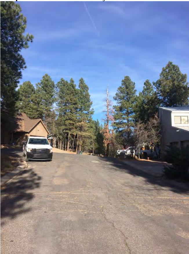
Photo No. 3: Advanced block cracking on Canyon Terrace Drive
