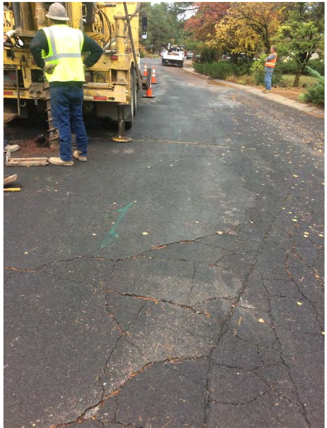
Photo No. 4: Transverse crack and alligator cracking on David Drive
