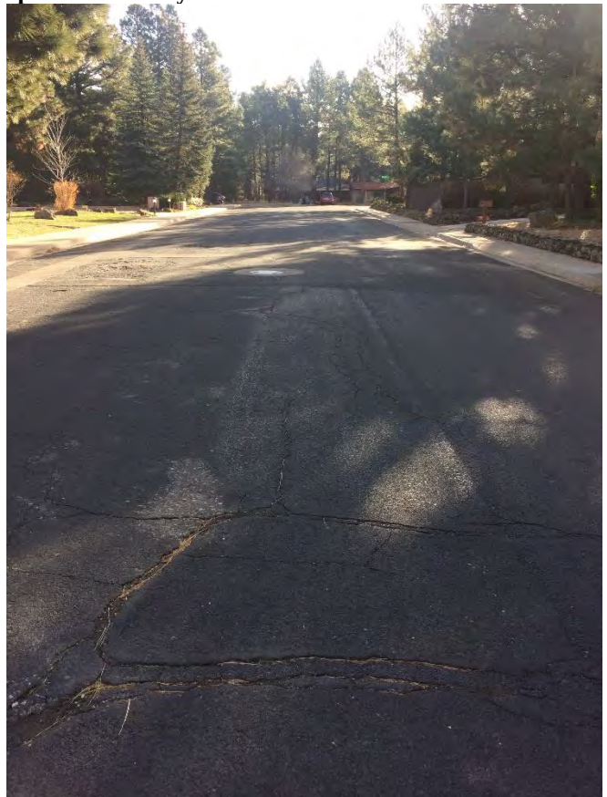
Photo No. 4: Transverse cracking on Hutcheson Drive
