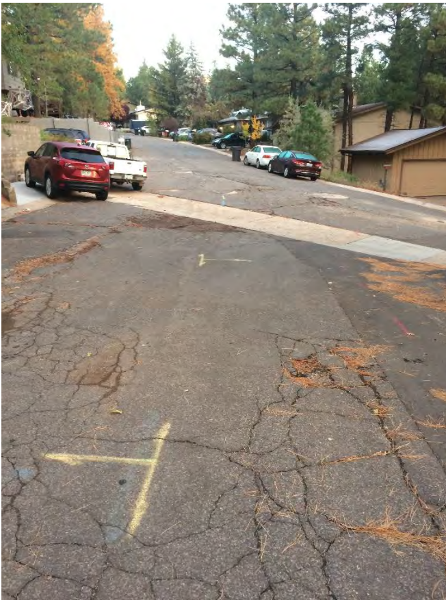
Photo No. 1: Alligator cracking, utility patching, and loss of asphalt wear surface on Canyon Terrace Drive
