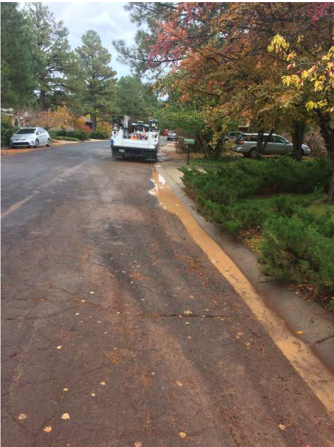
Photo No. 3: Alligator cracking and trench failure on David Drive
