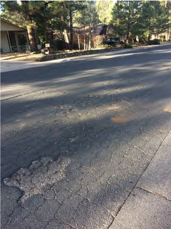
Photo No. 1: Alligator cracking on Hutcheson Drive
