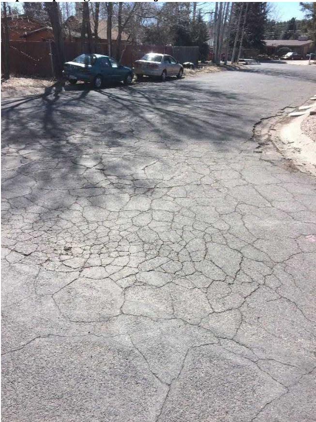
Photo No. 3: Severe alligator cracking on N. Navajo Dr.
