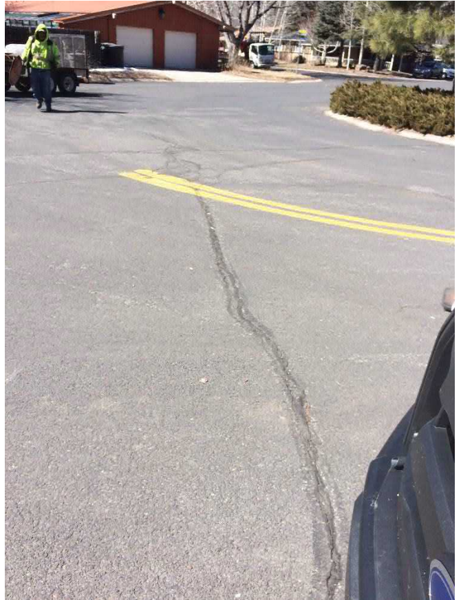
Photo No. 2: Block cracking on N. Talkington Dr.
