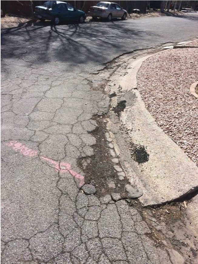
Photo No. 1: Alligator cracking, corner erosion and Asphalt spalling on N. Navajo Drive
