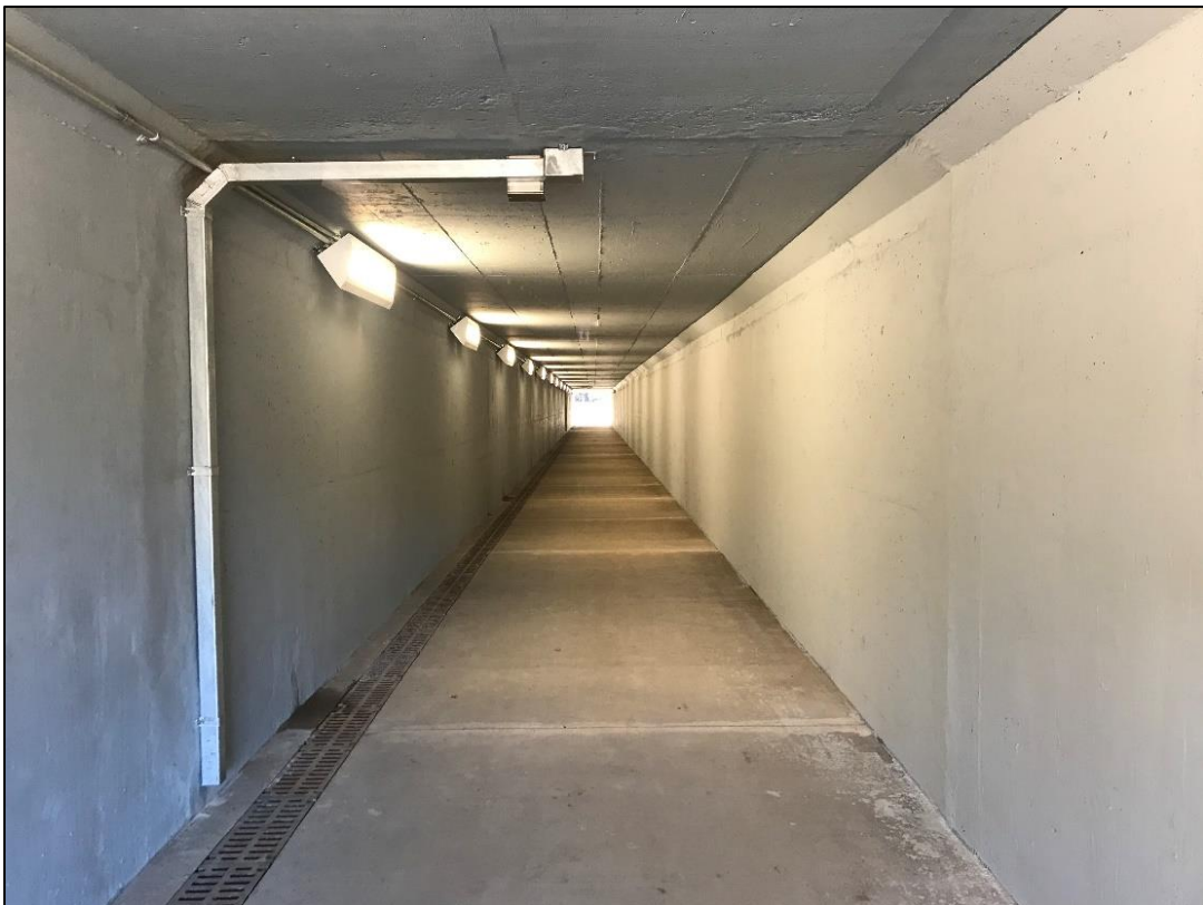
Looking west through the tunnel. Note the interior lighting and heated weep drain frost protection conduit.
