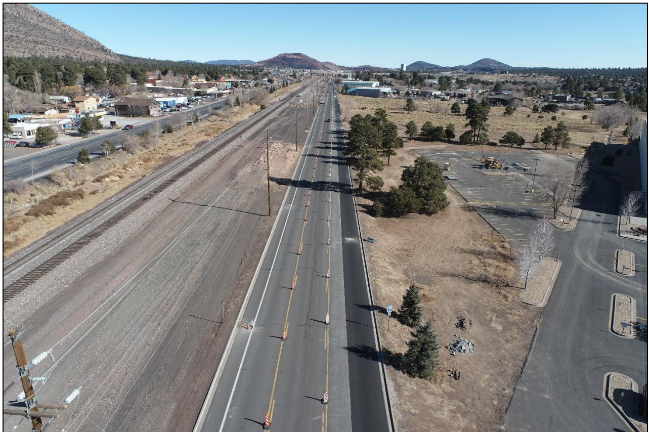
Industrial Drive ready for striping and valve adjustments, Industrial Dr. looking east
