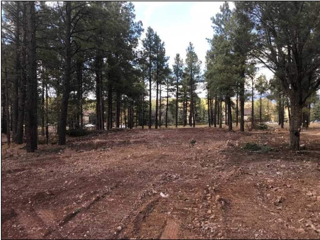
Former Fresquez buildings have been demolished and removed. Pictured above is where the former residence was located.
