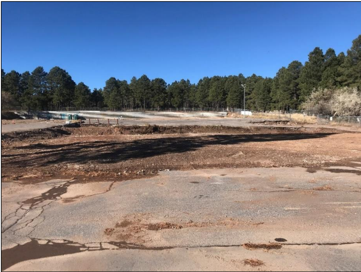
Former ADOT buildings have been demolished and removed. Photo taken looking west from Milton Rd. and University Dr. intersection.
