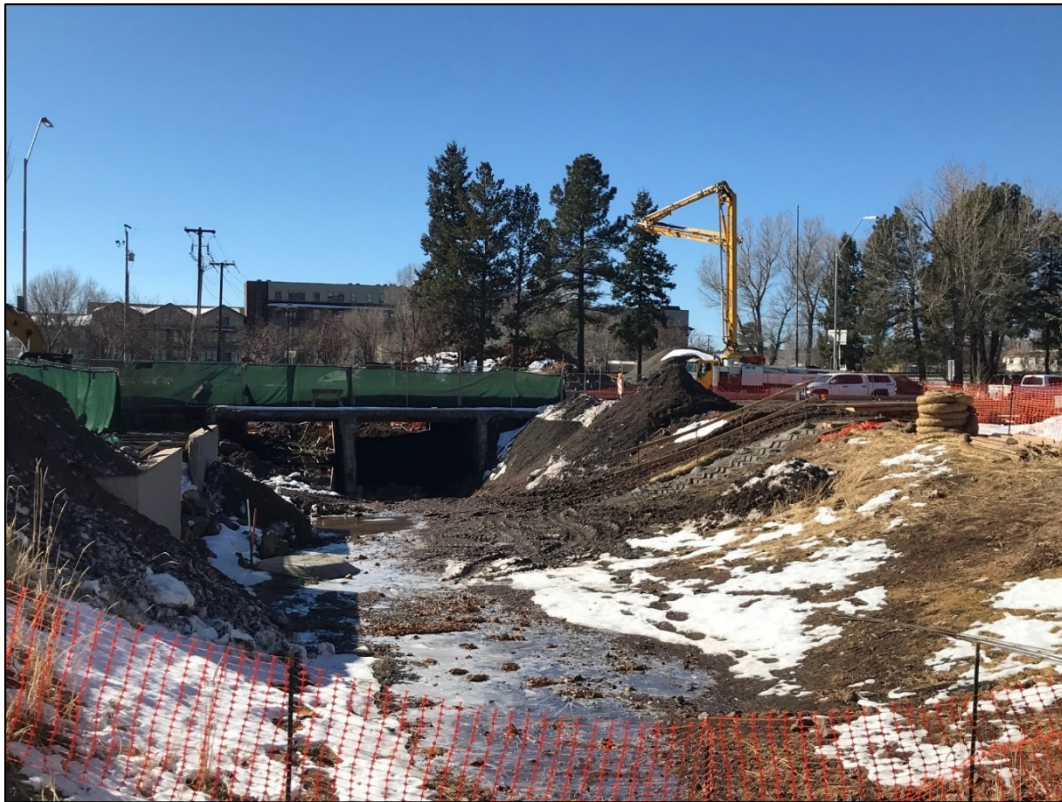
Backfill complete on the north side of the Rt. 66 and concrete placement of the southwest wingwall
