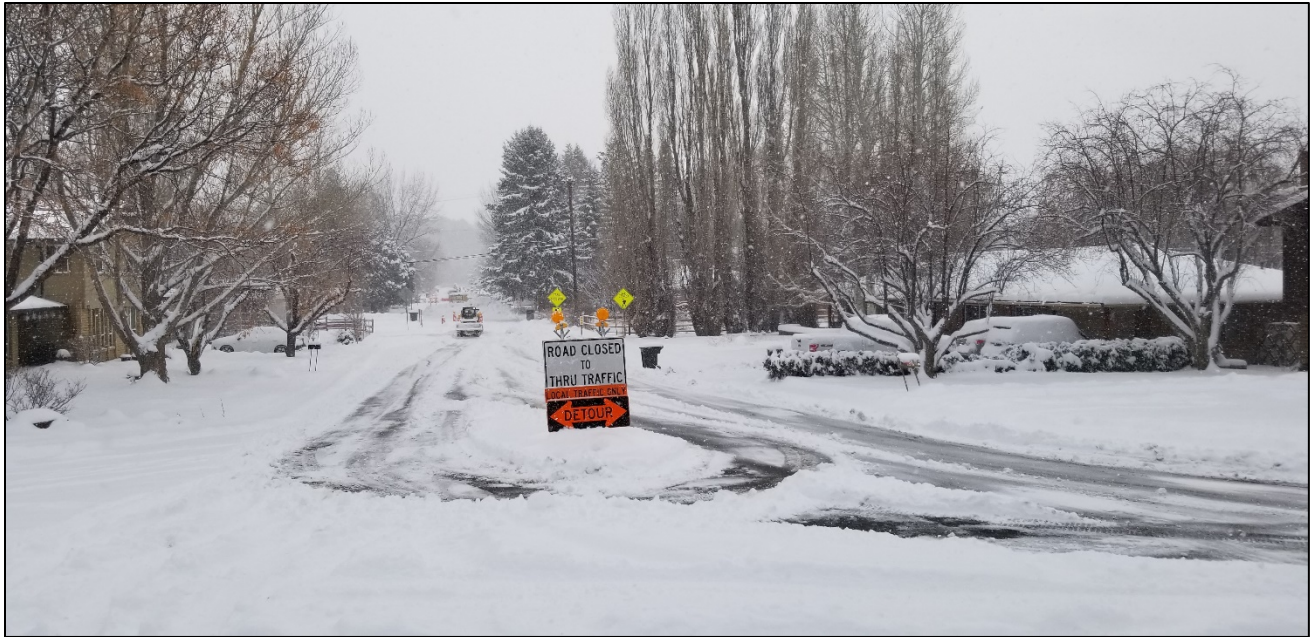
Beal Rd. / Aztec St. intersection looking east at the snow removal operations within the closure area on Beal Rd.
