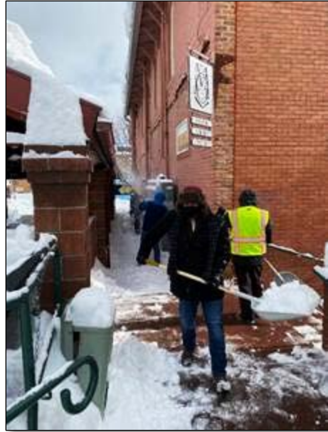
Clearing snow - parking garage canopy
