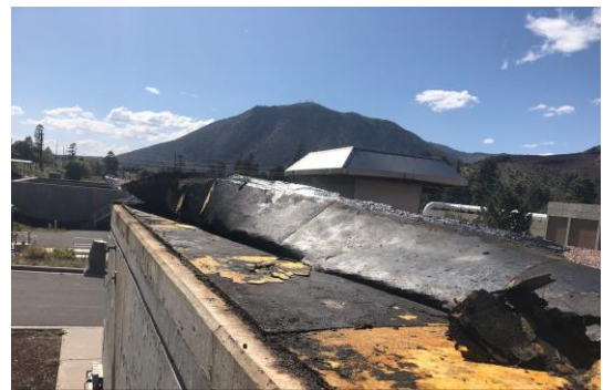
Wind damage to Wildcat Hill roof
