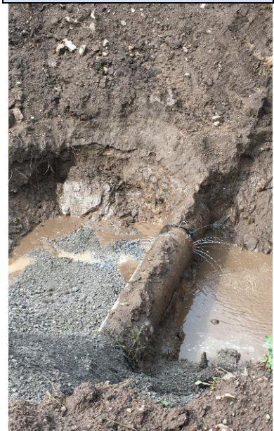
Inner Basin Pipeline break
