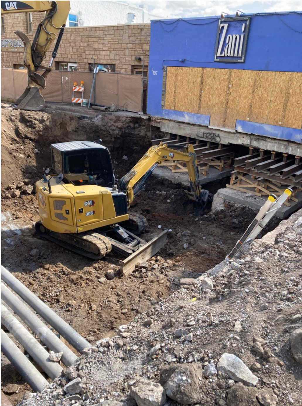
Phoenix Avenue Bridge, looking south at completed demolition and start of soil excavation to bedrock
