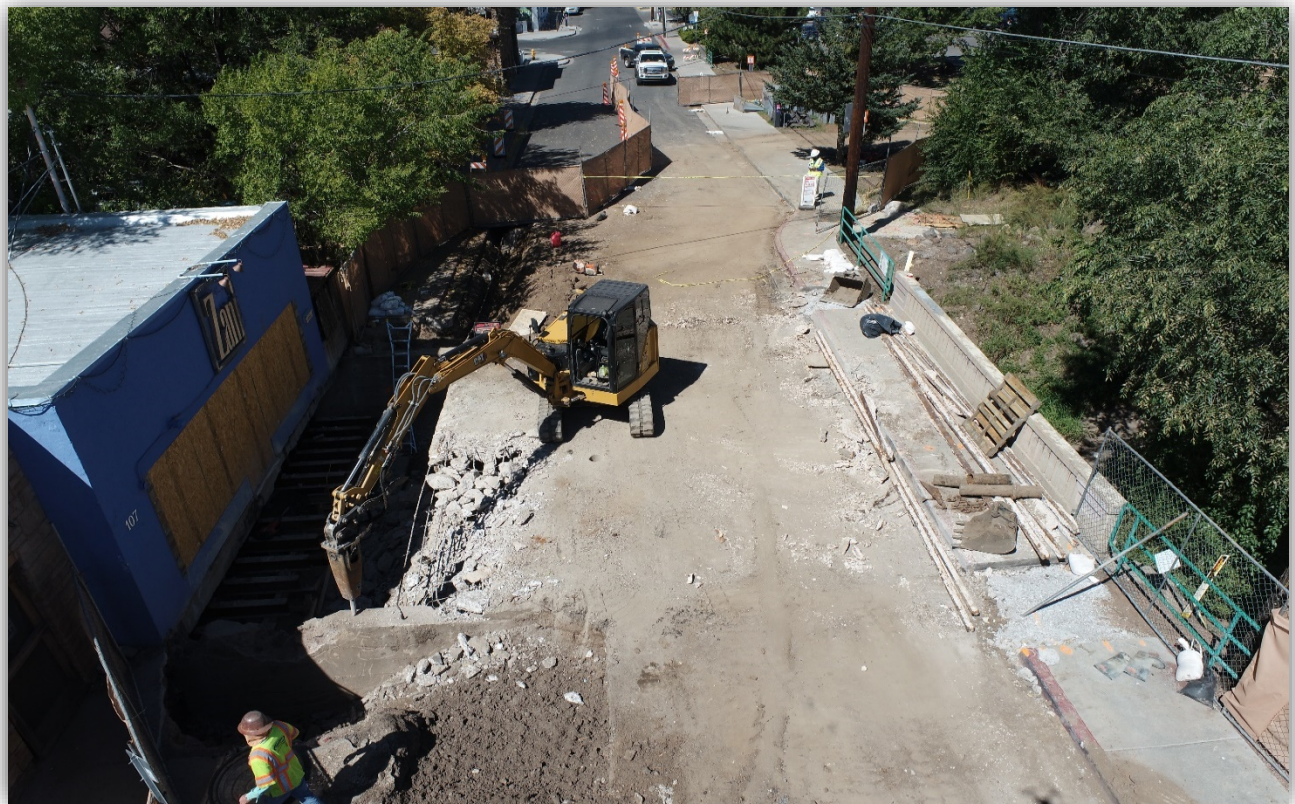
Phoenix Avenue Bridge, looking west at demolition of the existing bridge structure
