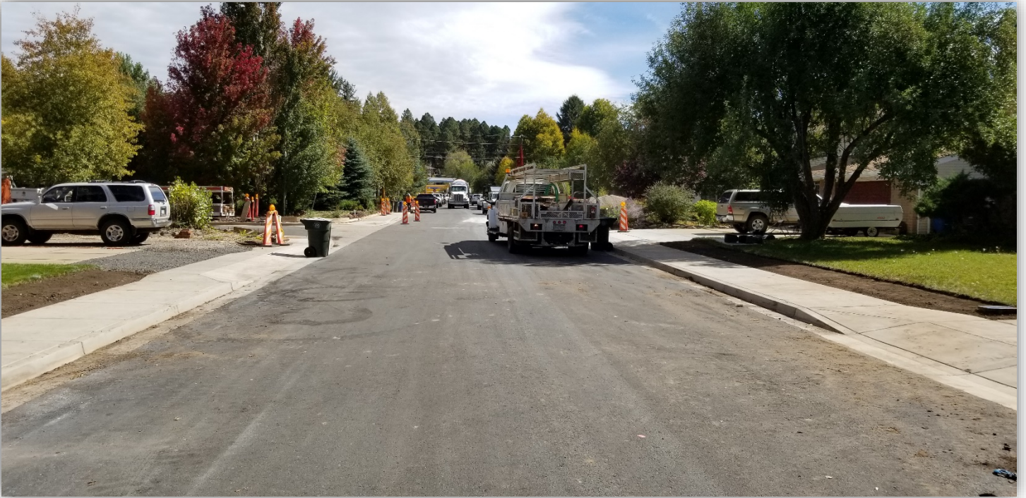
Beal Rd. west of McMillian Rd., looking east at final concrete and landscape restoration operations.
