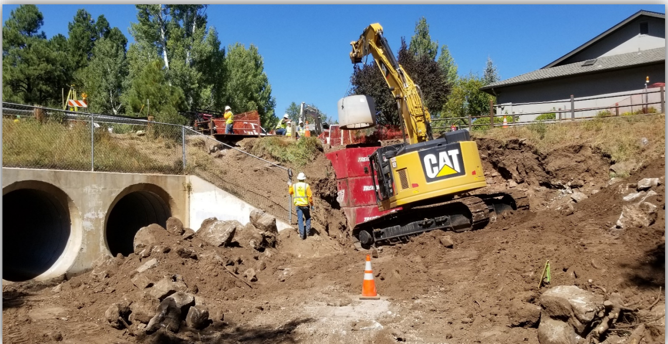
Crescent Dr. and Rio de Flag, looking north at the new sewer main installations connecting Crescent and Rio de Flag sewer mains.
