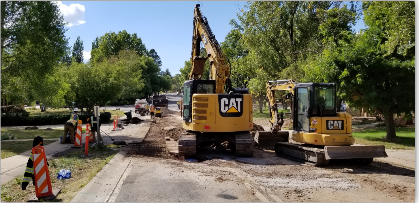
Beal Rd. west of Rio de Flag, looking west at water main and service installations.
