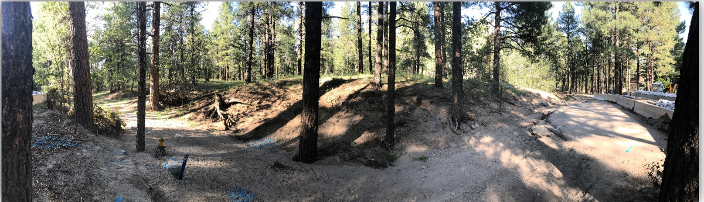
Pre-Construction Image of Channel Widening Project at North End of Paradise Road.
