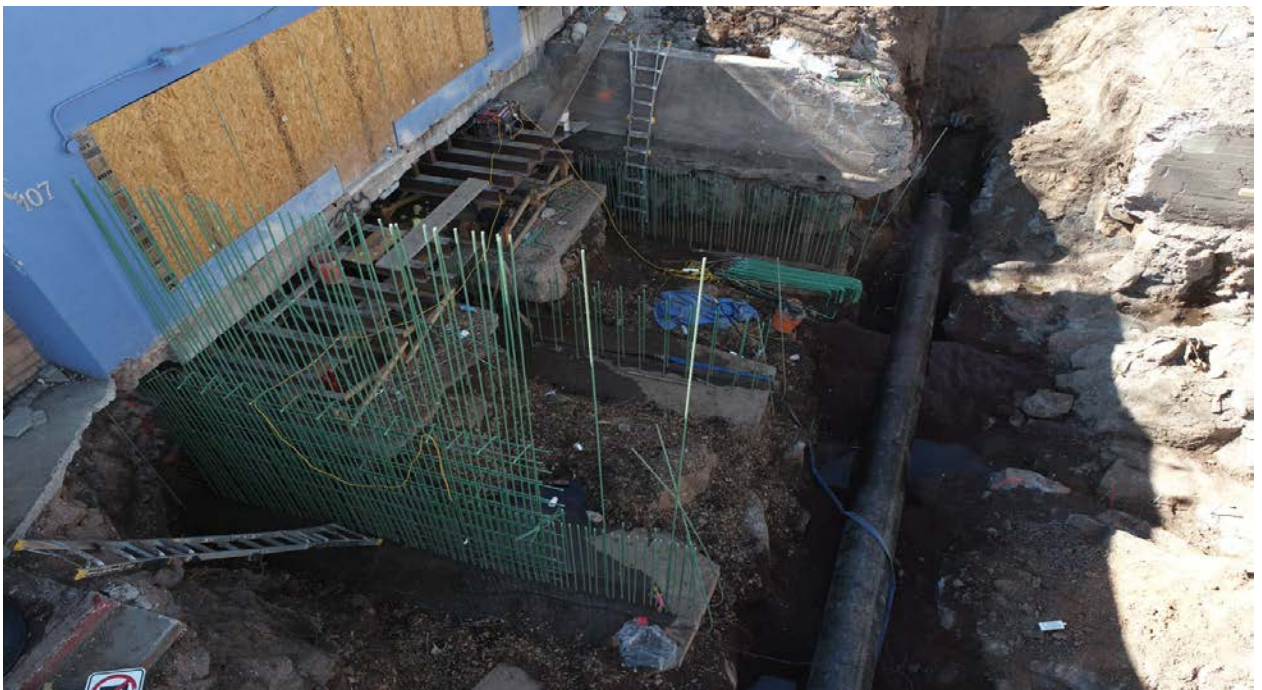
Phoenix Avenue Bridge, looking at the start of rebar placement for the new walls and installation of the steel casing for the new waterline.
