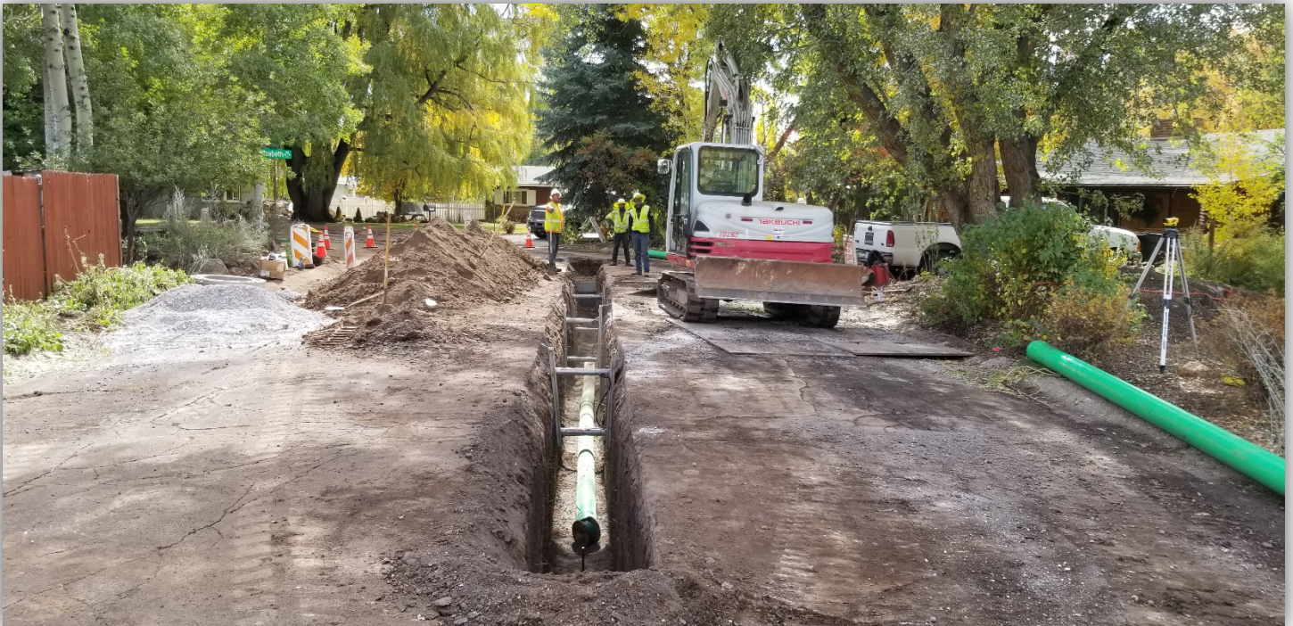
Navajo Dr. and Elizabeth Rd. corner, looking south at sewer installations on Navajo.
