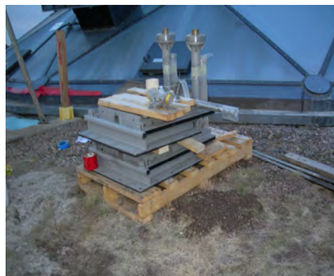
New Stainless Steel valves
