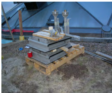
New Stainless Steel valves
