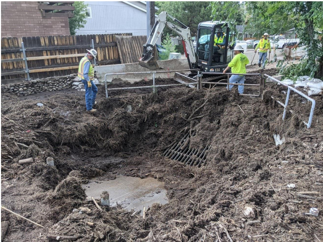
Figure 7: Emergency crews clean up debris from flash flooding in east Flagstaff on July 14th, 2021. Source: Flagstaff City Government.
