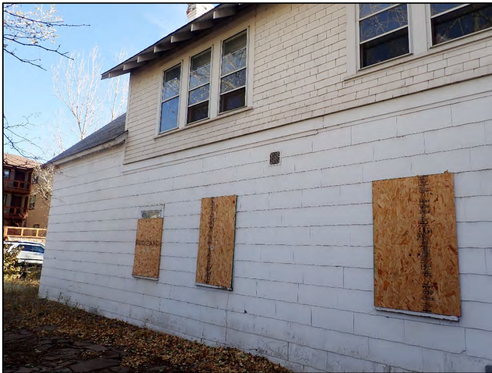
Figure C-30. Detail of the north elevation, showing the boarded-up windows on the first floor and the windows of the sleeping porch above.
