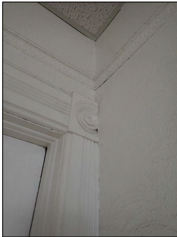
Figure D-64. Alternative view of the other upper corner of the door jamb and picture molding in the sitting room.
