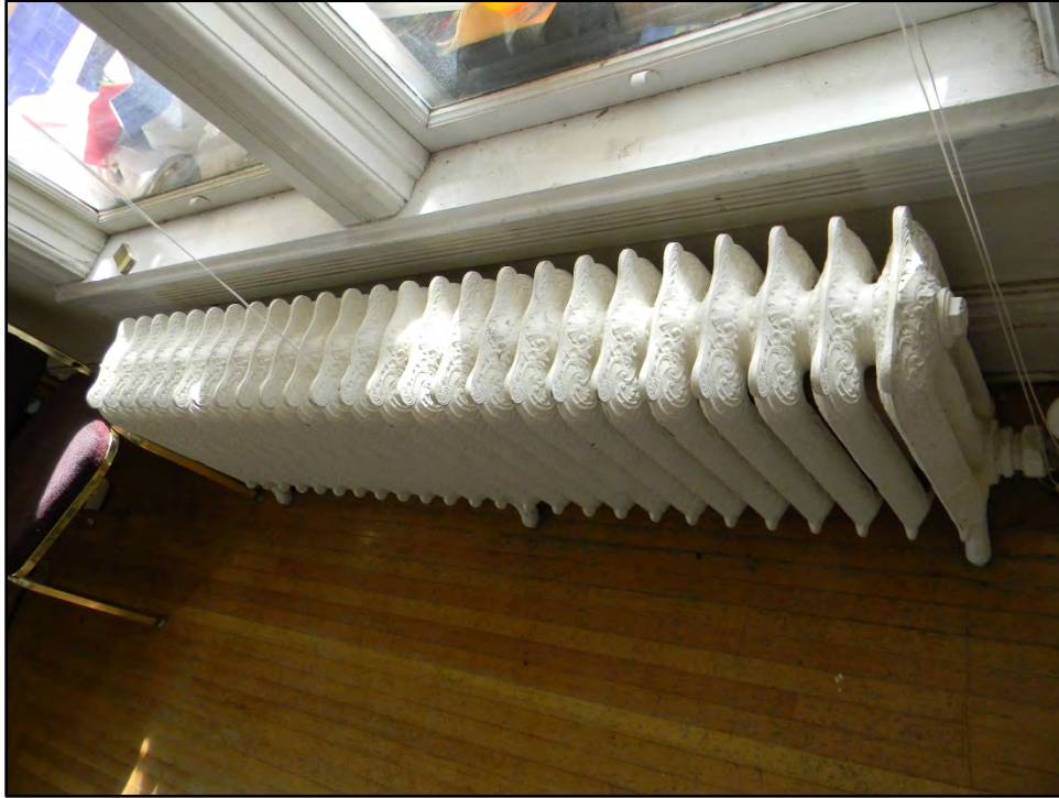
Figure D-69. View of the decorative radiator still present in the sitting room.
