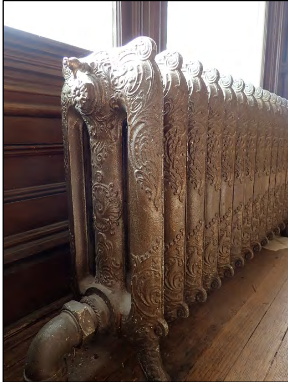
Figure D-101. Detail of the decorative radiator.
