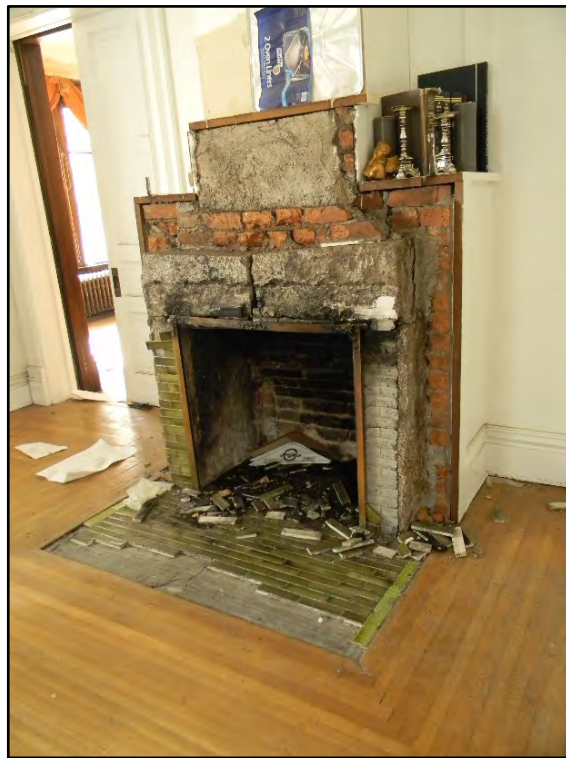
Figure D-72. Overview of the deteriorating fireplace in the sitting room.
