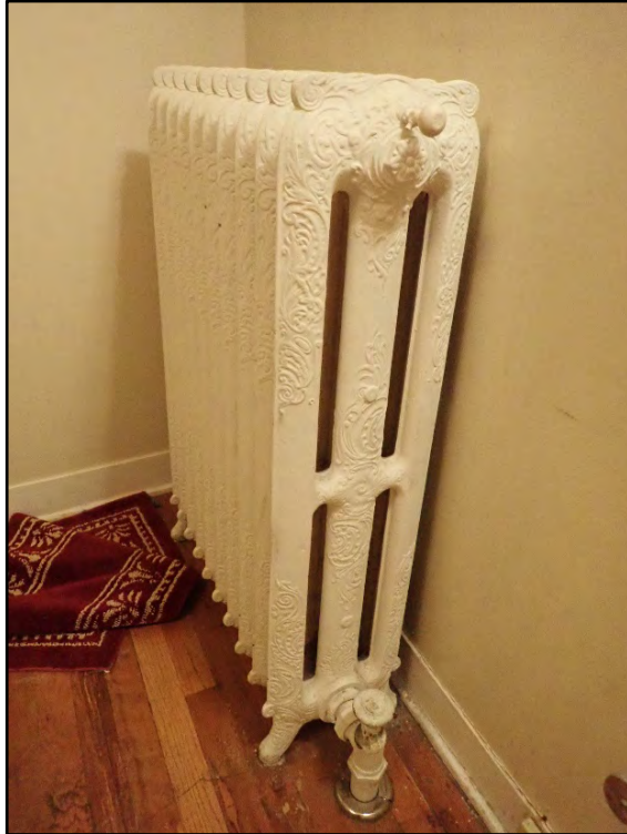
Figure D-191. Detail of the decorative radiator in the bedroom.
