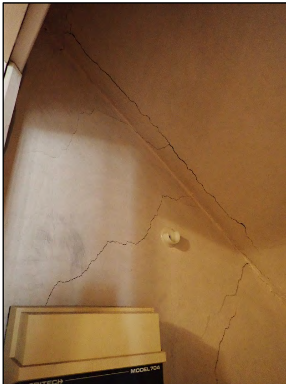
Figure D-226. Detail view of the lath-and-plaster construction of the walls in the under-stair closet, which are cracking.
