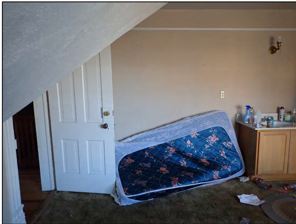
Figure D-372. A view from the gable cut in the second bedroom, with the original bedroom door and picture molding that encircles the room.
