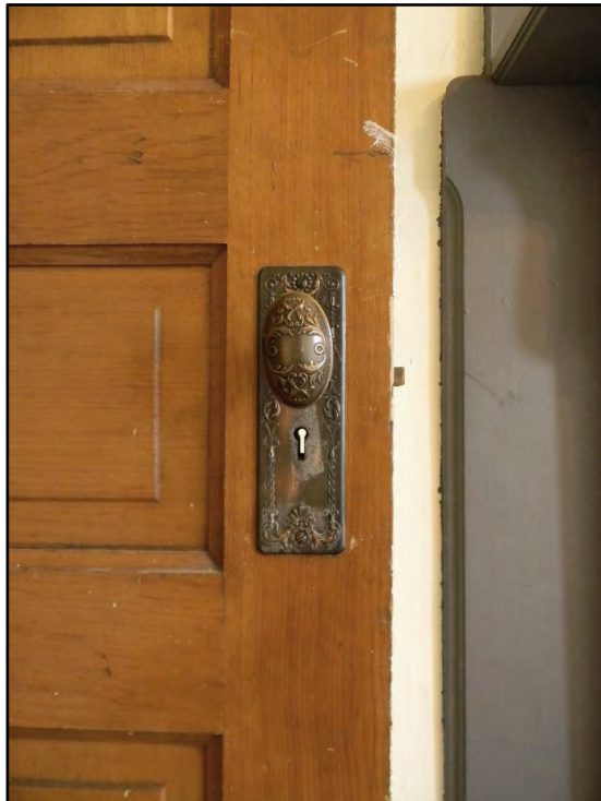
Figure D-252. Close-up of the original door knob and rose affixed to the solid-core wood door.
