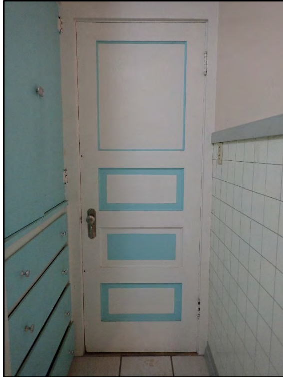
Figure D-303. The interior of the bathroom door to the east side hallway.
