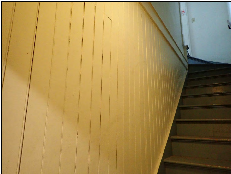
Figure D-326. The batten paneling in the secondary stair to the second stair, which was likely reserved for family use.
