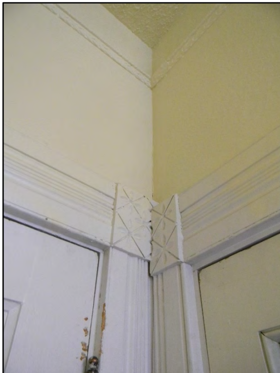
Figure D-264. Close-up of the picture molding above the wood details of the door trim in the first small bedroom.
