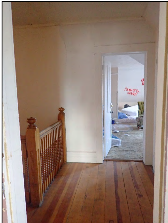
Figure D-356. View back into the main hallway, with the second bedroom beyond (note the extensive cracking in the walls and ceiling in this part of the hallway).
