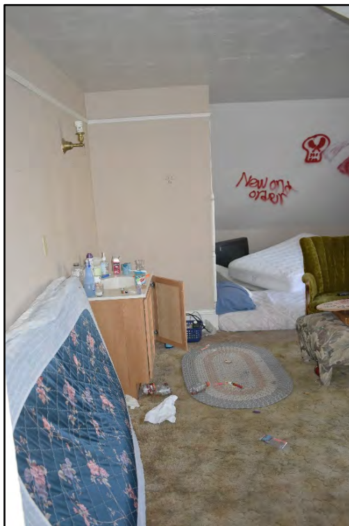
Figure D-366. Walking into the second bedroom reveals extensive graffiti due to squatters that broke into the residence.
