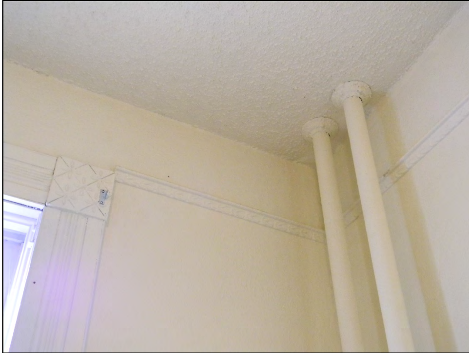
Figure D-257. Detail of the decorative window trim, picture molding, and pipes in the small bedroom.
