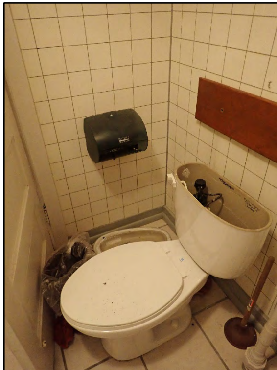
Figure D-284. The toilet in the small hall bath (the door is open in this image).
