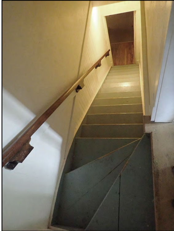
Figure D-337. View down the secondary stair as seen from the second floor.
