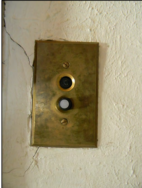
Figure D-355. Close-up view of the historic-era light switch and brass faceplate in the bedroom.
