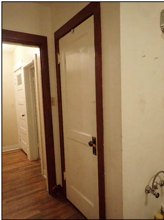
Figure D-314. A view of the closet door in proximity to the hallway.
