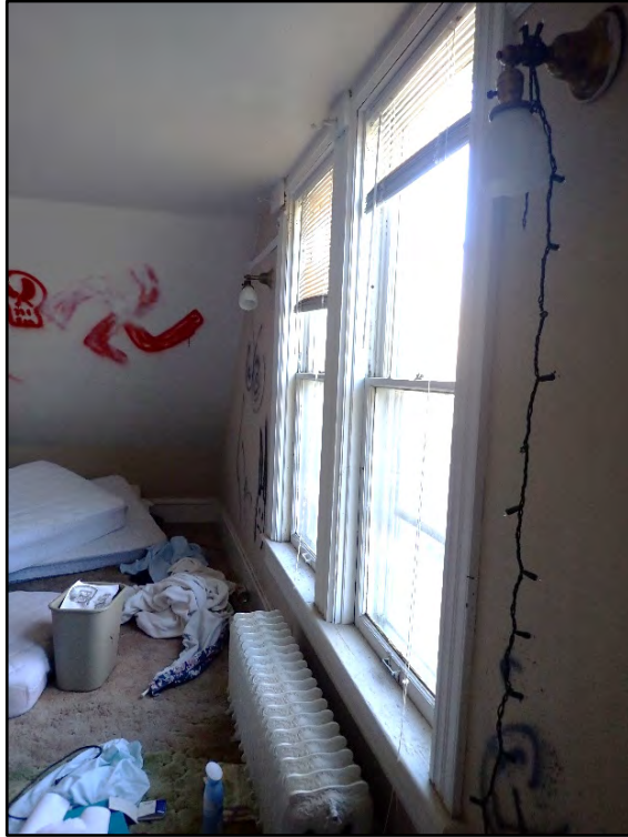
Figure D-375. An oblique view of the original windows in the second bedroom.
