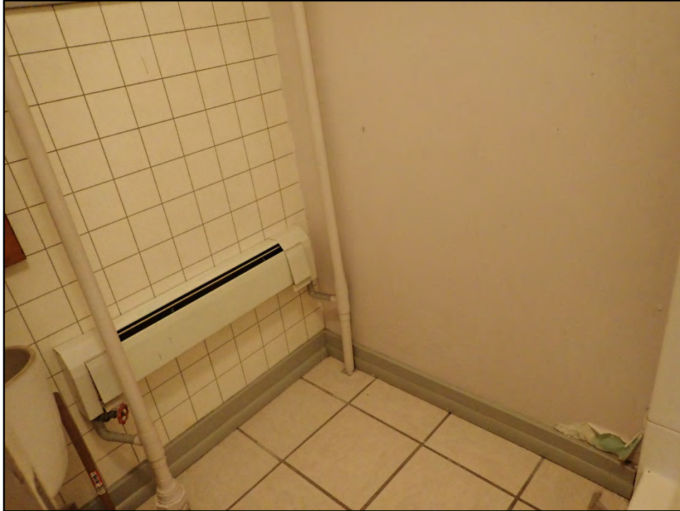
Figure D-283. A small heater, with modern tile floor and wall juxtaposed with the original historic-era finish of the wall on the right.
