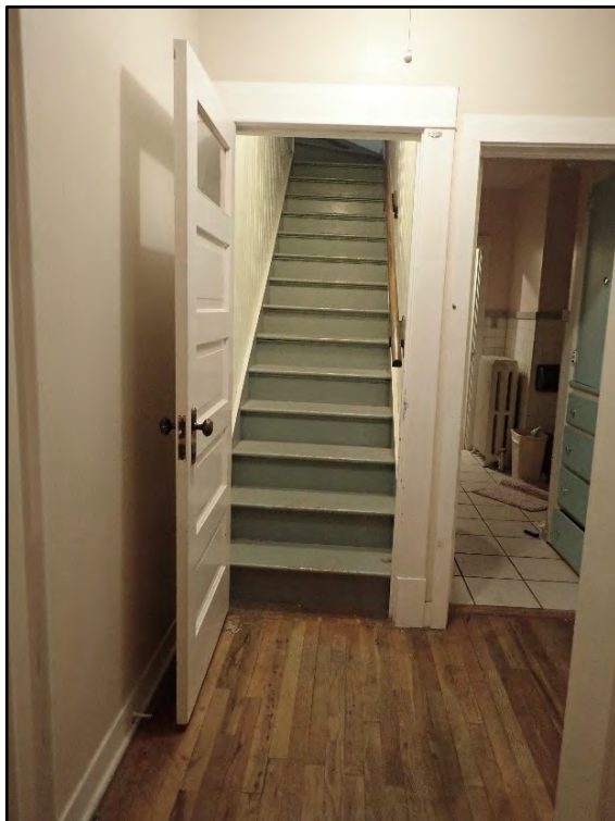
Figure D-322. The original door of the secondary stair to the upper floor.
