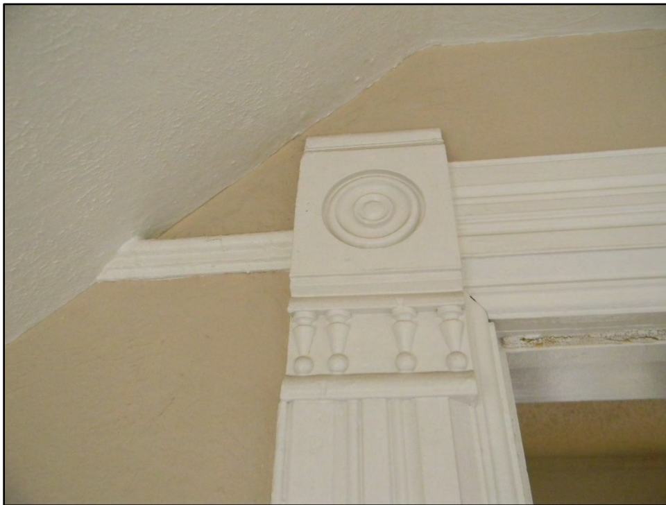
Figure D-370. A close-up view of the most ornate architrave and corner blocks in the residence (note the picture molding).
