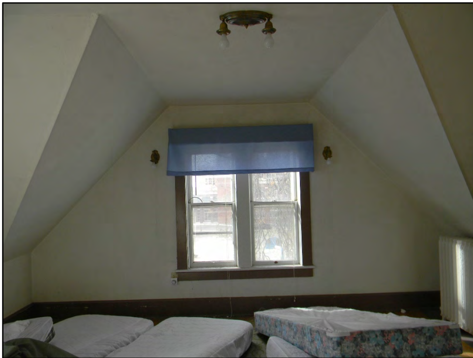
Figure D-346. View of the south gable end of the first bedroom.
