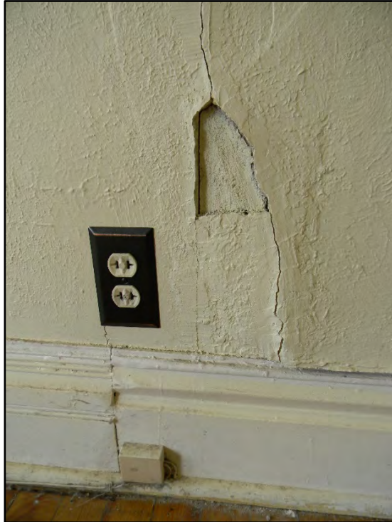
Figure D-251. Close-up view of the cracked plaster wall finish (which was once an open door to the entrance hall, as indicated by the difference in baseboards).
