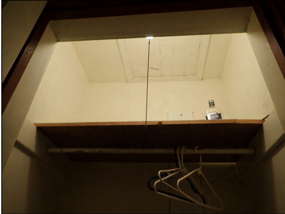
Figure D-317. The upper portion of the closet of the third small bedroom.
