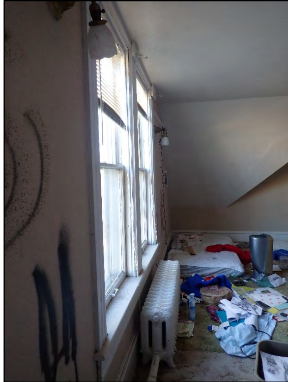
Figure D-379. An alternate view of the other side of the windows in the gable end facing the south end of the room.
