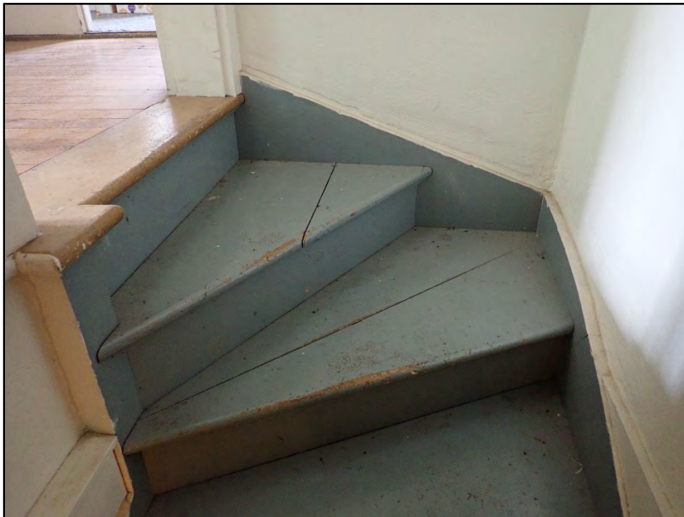
Figure D-334. A detailed view of the 90-degree winder of the secondary staircase.
