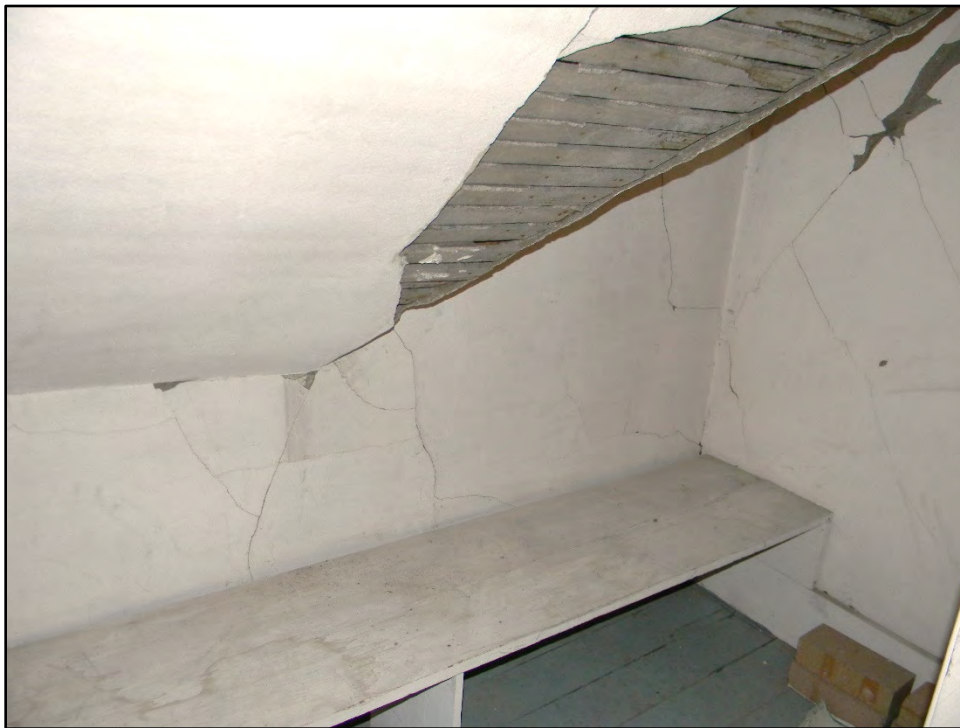
Figure D-364. An alternative view of the interior of the storage closet, the doors of which likely served to hide what would have been an awkward wall space.
