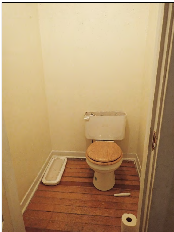
Figure D-274. A toilet has been installed in the second small bedroom.
