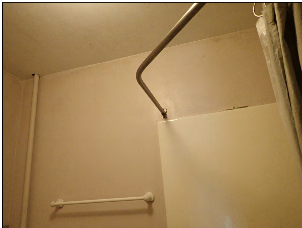
Figure D-282. A modern stand-alone shower with other modern fixtures as seen in the hall bath.
