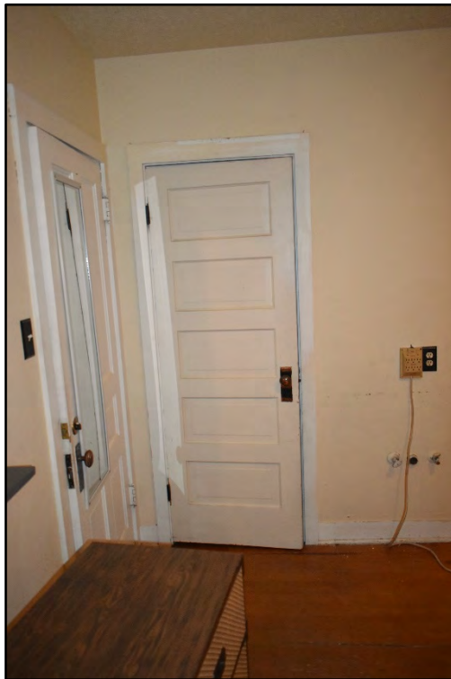
Figure D-272. The small closet with solid-core wood door in the second bedroom on the first floor.
