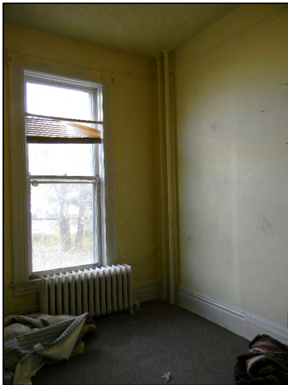
Figure D-256. View of the window and radiator of the first small bedroom.
