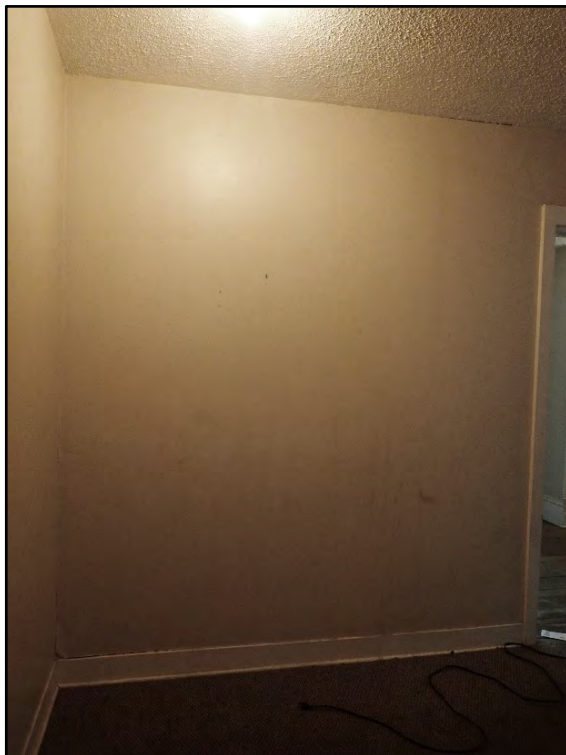
Figure D-276. A view of the corner of the hallway to the bedrooms on the first floor.
