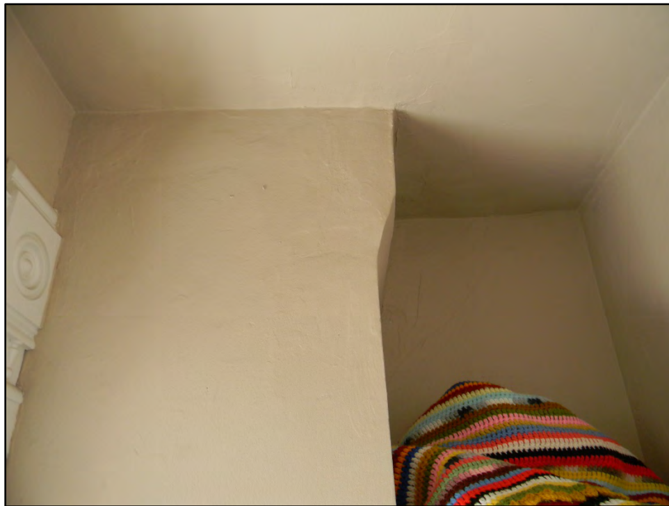
Figure D-386. A close-up view showing the workmanship of the connected closet, which made use of even the tightest of spaces resulting from the chimney.
