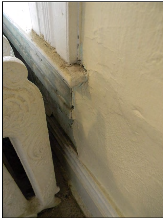
Figure D-258. Close-up view of the damage around and under the window.
