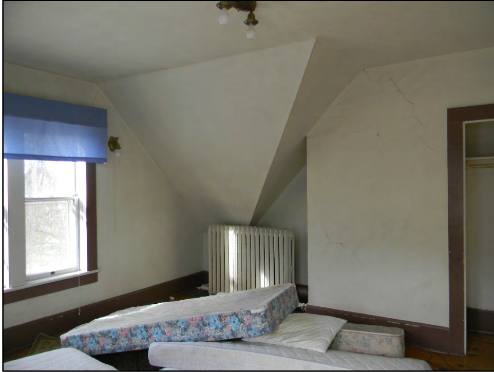
Figure D-347. The edge of the gable cuts into the room (note the cracked wall at right).
