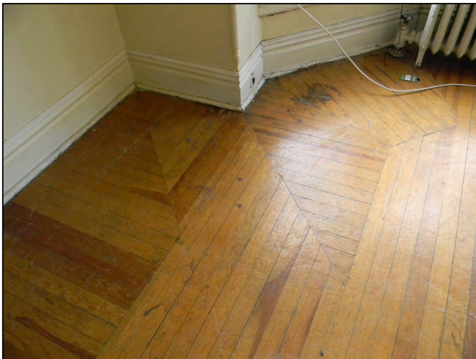
Figure D-250. View showing the patterned hardwood floors in the master bedroom, reminiscent of the sitting room but distinctly more intricate.
