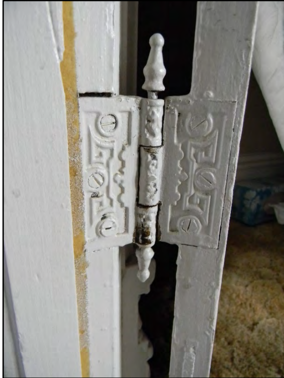
Figure D-369. A close-up view of another late nineteenth century brass door hinge.
