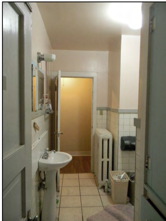
Figure D-296. A view through the connected bath to the opposite hall (toward the fourth small bedroom and chapel).
