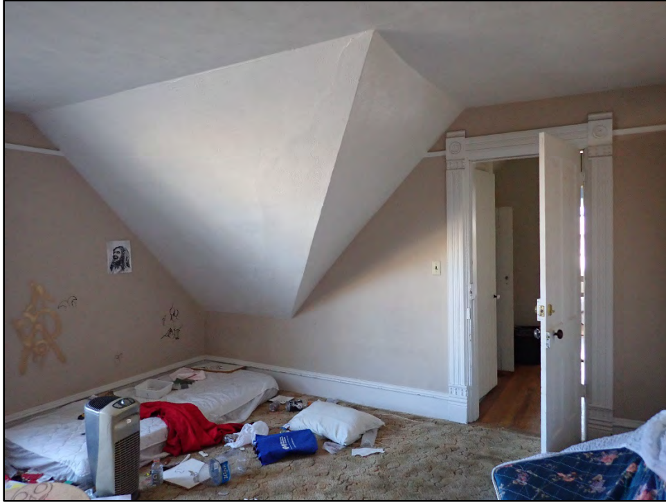
Figure D-381. The roof substantially cuts into this room due to the gable design (note the modern carpet, which hopefully protects original hardwood floors below).
