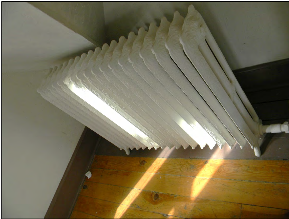
Figure D-352. A decorative radiator, similar to those throughout the residence, sits under the roof which cuts in because of the gable end.
