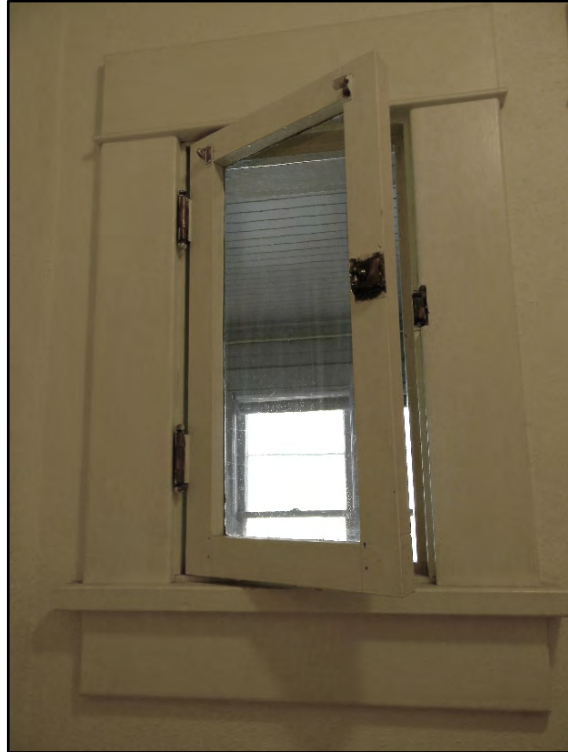
Figure D-445. A detail view of the small casement window and oversized wood trim.
