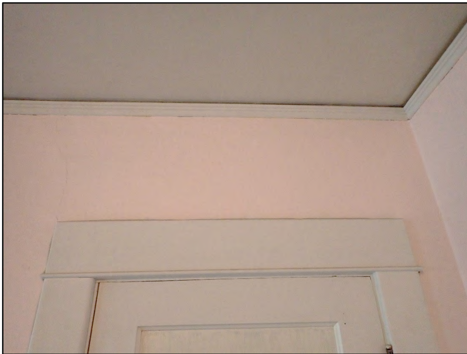
Figure D-438. Detail of the wood door trim as well as the upper molding which is indicating the ceiling may be separating from the walls.
