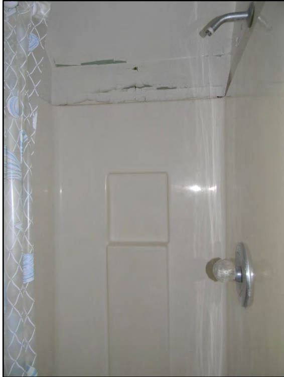
Figure D-525. Detail view of the separate shower that now fills in the space between the modern bath and large bath.
