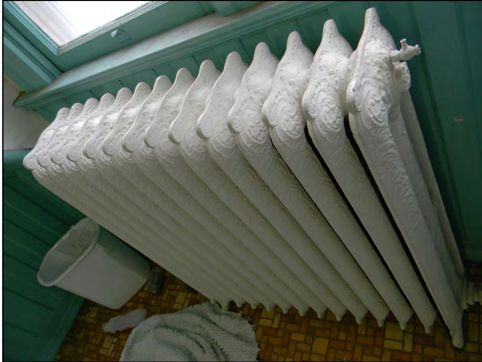
Figure D-535. The large radiator under the paired windows of the large bath.
