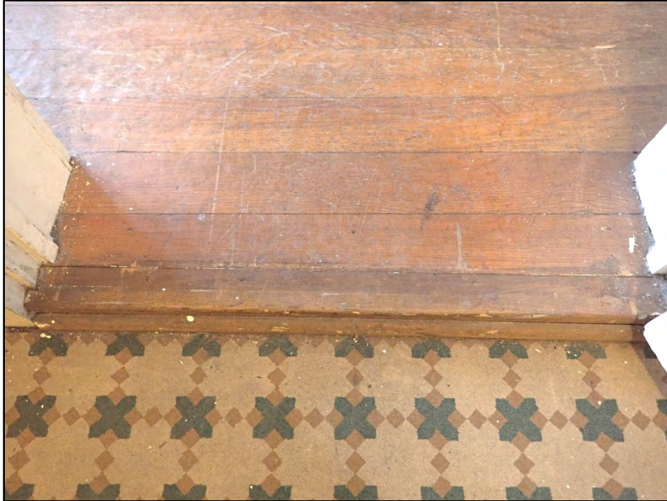
Figure D-453. A close-up view of the historic-era linoleum and original hardwood floors between the third bedroom and laundry room on the second floor.
