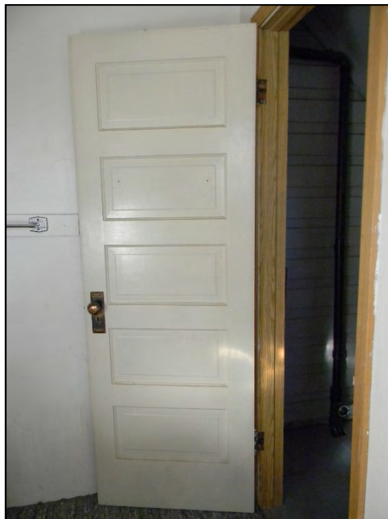
Figure D-494. A repurposed door fit into the modern sheetrock/drywall construction that closes off a small storage area behind the tub/shower.
