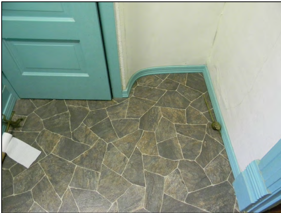
Figure D-516. A detailed view of the floor-wall junction of the same wall, also showing its curved design (the linoleum likely covers original hardwood floors).
