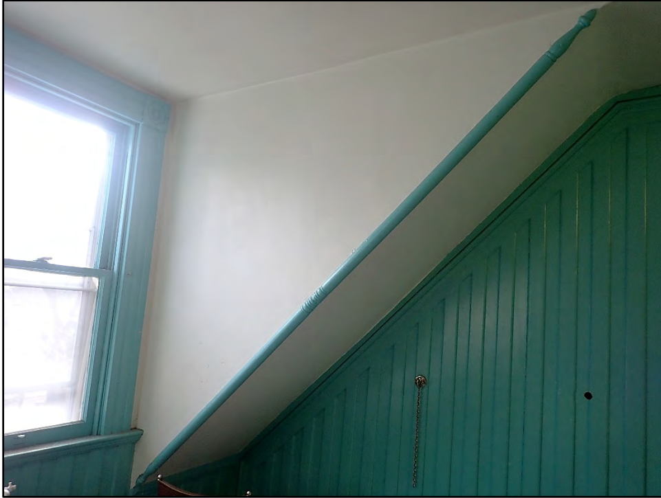
Figure D-533. Detail of the wood accent on the corner of the cut in of the ceiling formed by the framing of the dormer (which was constructed by 1901 and is seen in the 1906 photographs in Appendix B).
