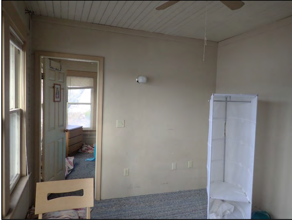
Figure D-481. An alternative overview of the interior of the second small room, looking back toward the first small room (note the modern drywall covering the original wood wall on the right).
