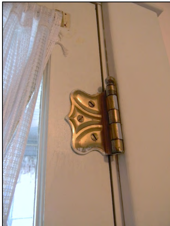
Figure D-428. A close-up view of the brass door hinges of the French doors.
