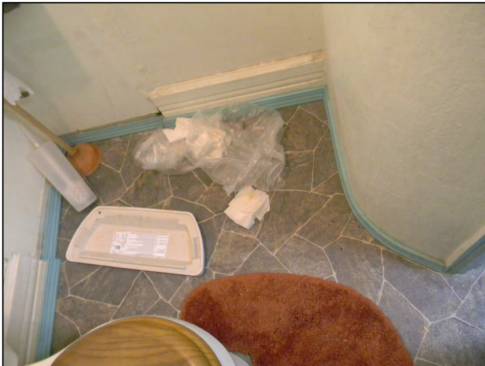
Figure D-518. Detail of the floor of the toilet area, showing the back of the curved wall (note the missing baseboard suggests this was reconfigured or renovated after it was completed).
