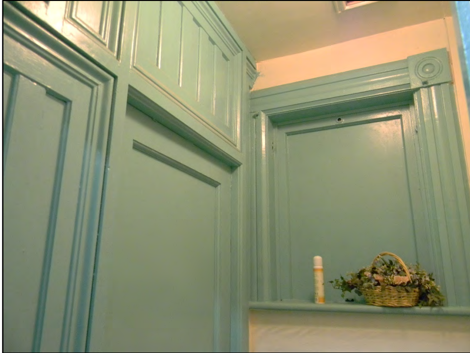
Figure D-519. Detail of the original window and door to the small toilet area that are now closed off (the shower room is on the other side of the door on the left and the modern bath is behind the small upper window).
