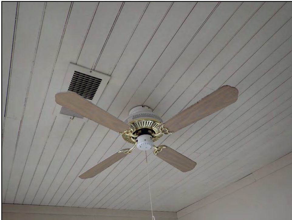
Figure D-482. Detail of the modern ceiling fan and heating register in the second small room.
