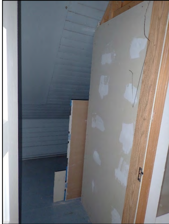
Figure D-495. The interior of the storage area reveals the modern drywall behind the tub/shower.
