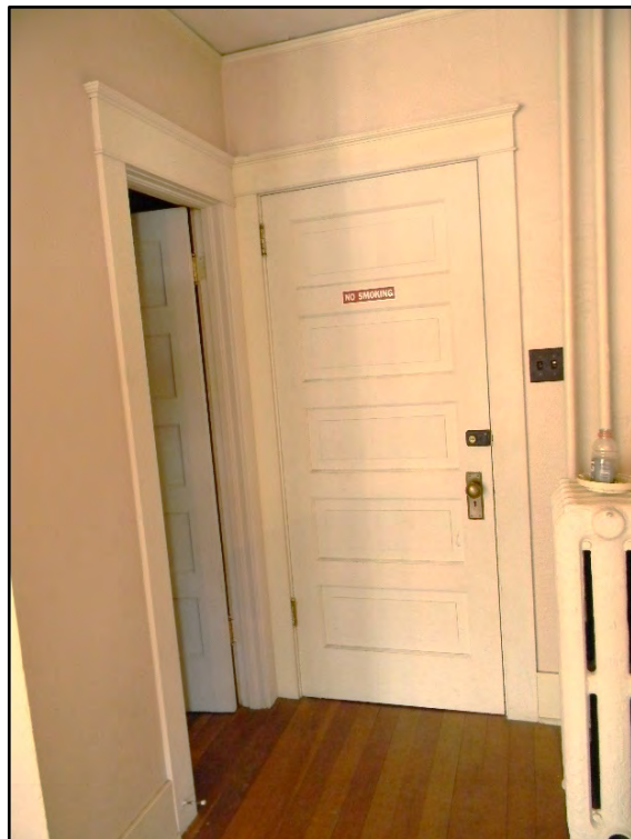
Figure D-398. Stepping back into the room, this view shows the orientation of yet another closet space in relation to the hall door.
