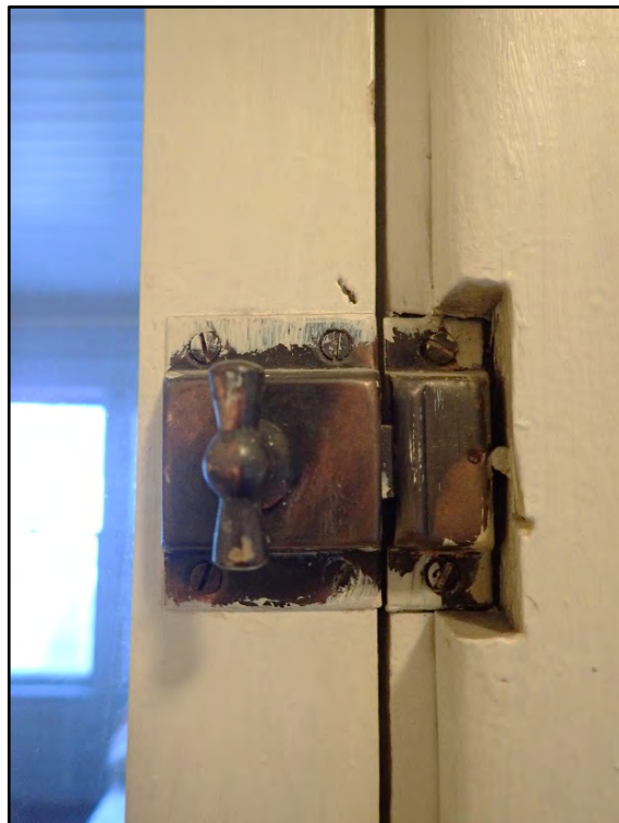
Figure D-446. A close-up view of the brass latch of the small casement window.
