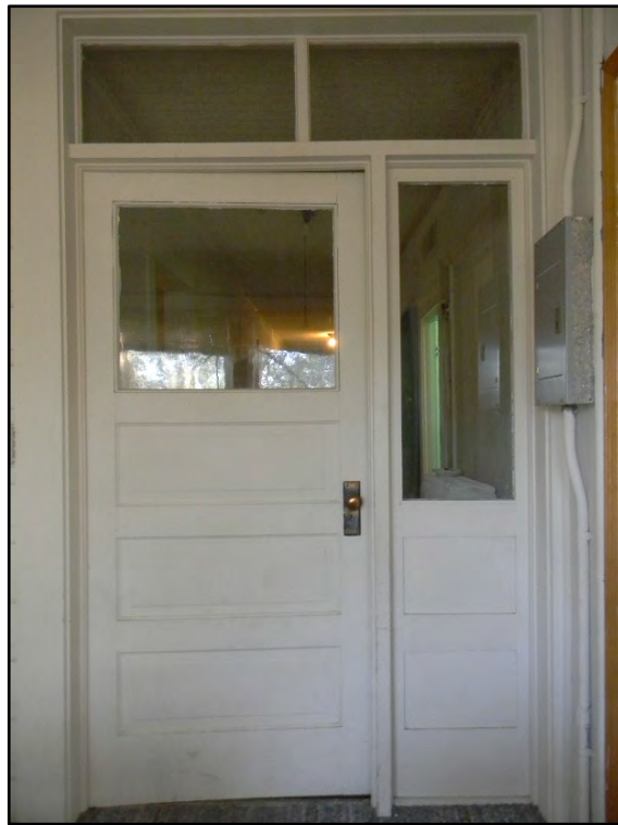
Figure D-504. Detail view of the once-exterior door that provided access to the sleeping porch that once stretched the length of the west side of the residence on the second floor.
