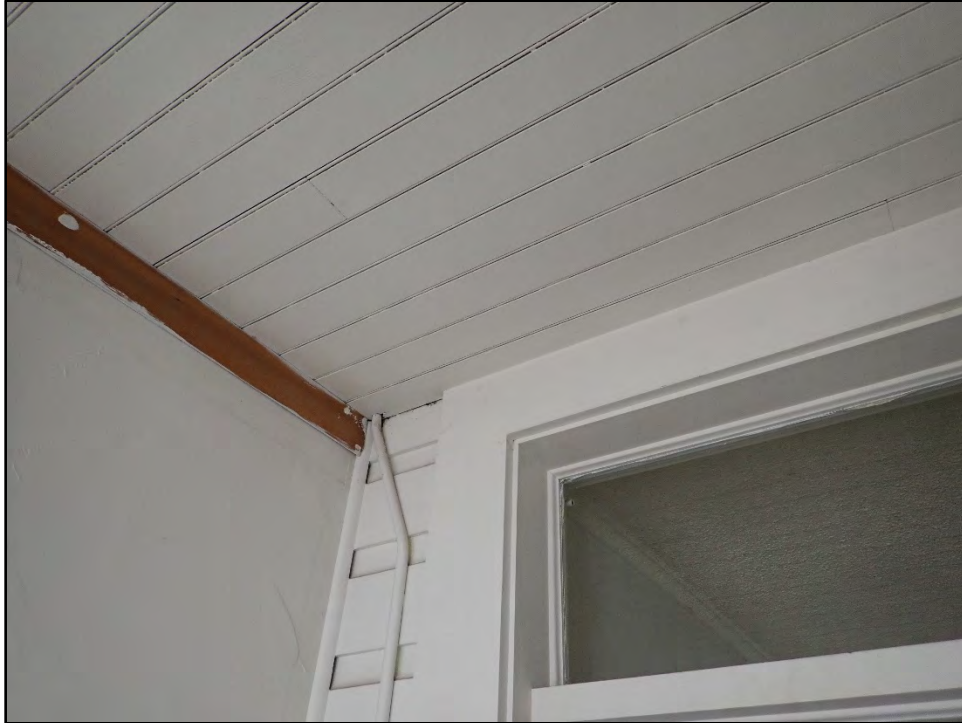
Figure D-505. Detail view of the original wood construction of the former sleeping porch (note the drop siding) with the modern drywall on the left.
