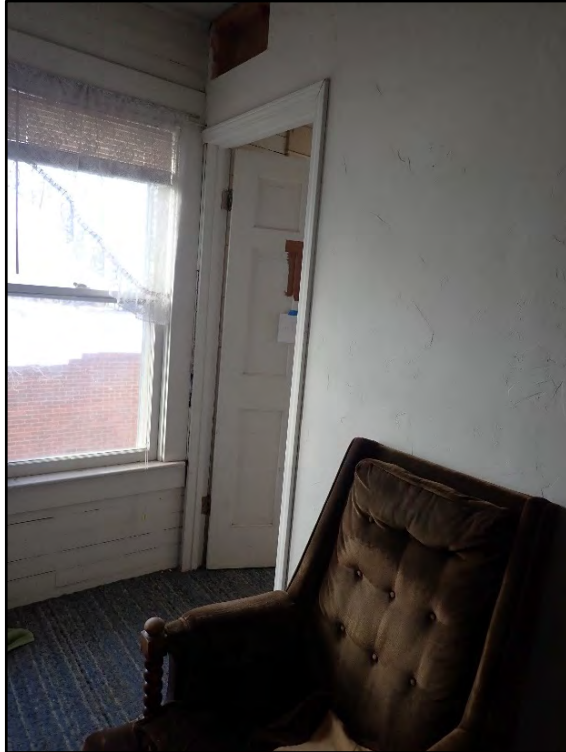
Figure D-485. A look back toward the door to the second small room, showing the modern sheetrock/drywall installed to divide up the former sleeping porch.
