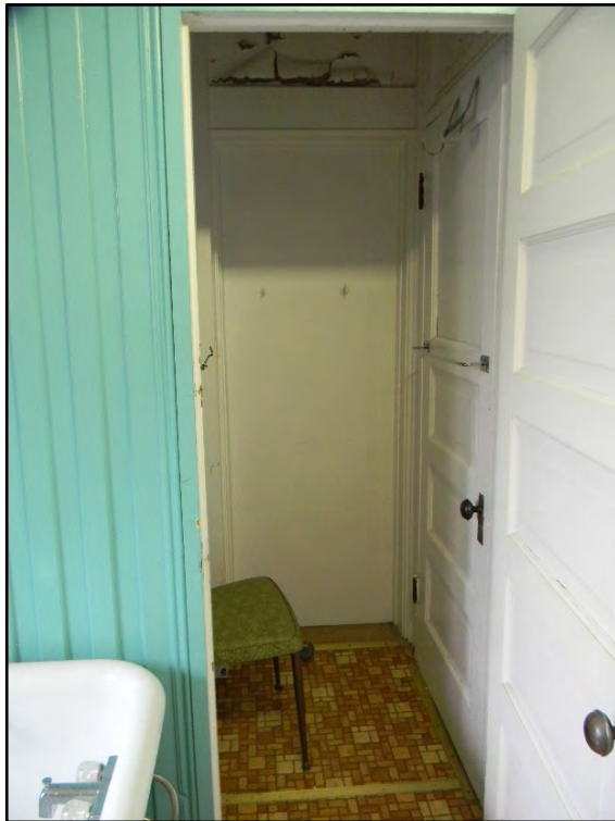
Figure D-524. The interior of the separate shower, showing yet another doorway that has since been closed off (also into the modern bath).
