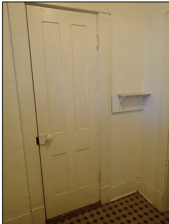
Figure D-450. The interior of the door to the third bedroom within the laundry room.
