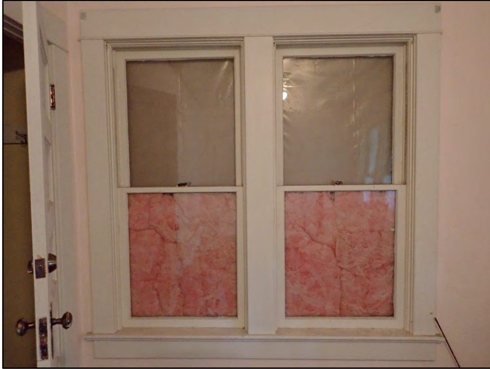
Figure D-433. A detailed view of the once-exterior windows that have been filled in with insulation and covered over with drywall.
