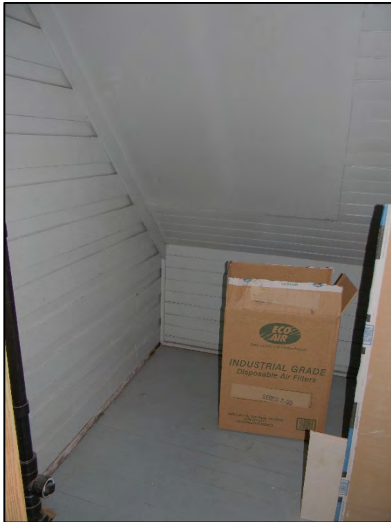
Figure D-498. The original drop siding and wood paneling of this small space, which is part of the construction completed between 1910 and 1916.
