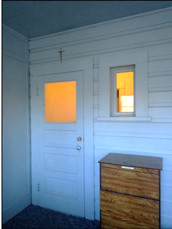
Figure D-455. The door and window of the laundry room as seen from the interior of the sleeping porch.
