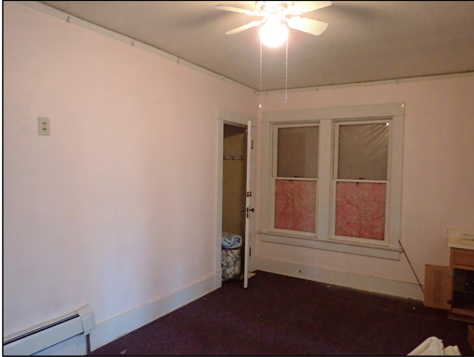
Figure D-423. An alternate view of the interior of this bedroom toward the corner closet.
