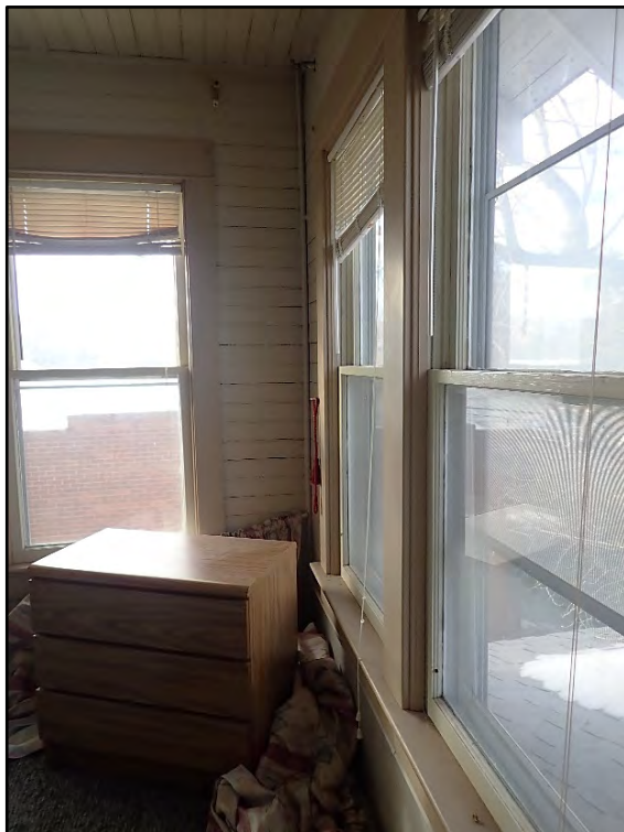
Figure D-470. View of the corner of the first small room on the second floor, created when this sleeping porch was divided into smaller spaces.
