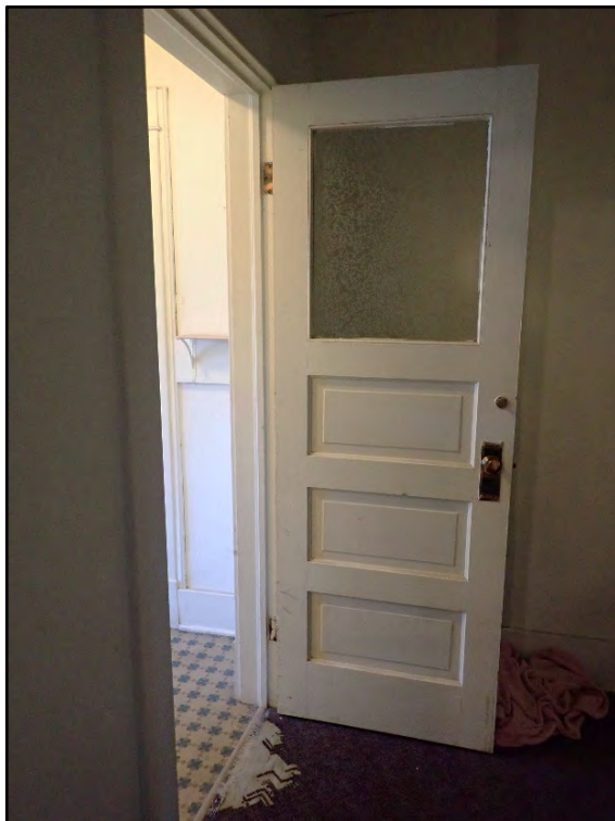
Figure D-440. The original wood panel door with privacy glass, suggesting this small space was once a bathroom.
