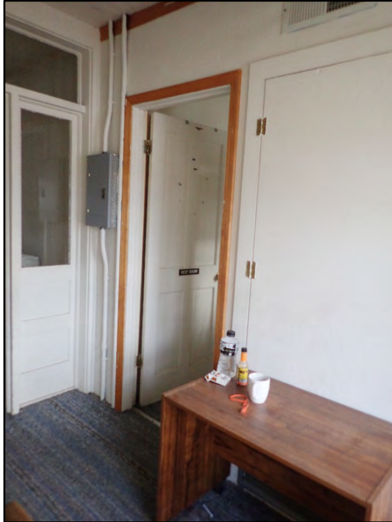
Figure D-487. View of the door to the modern bath with an upgraded electrical box next to it.
