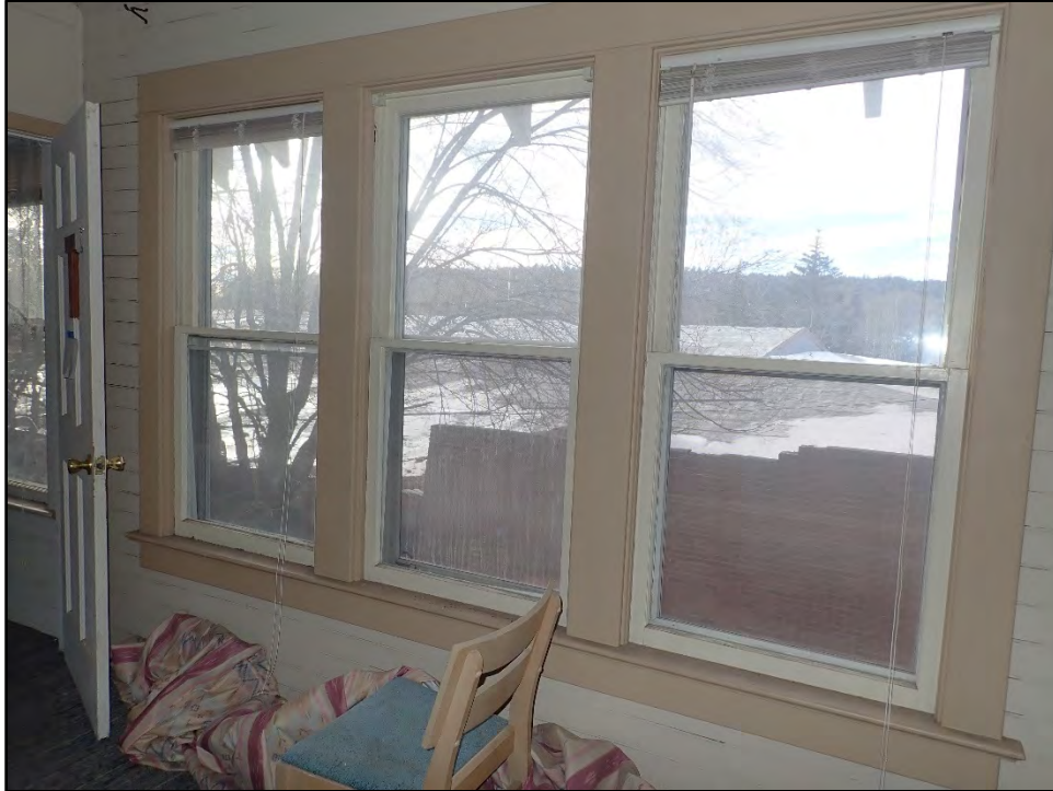
Figure D-479. View of the row of three original windows in this part of the former sleeping porch, with the midcentury Catholic school visible outside.
