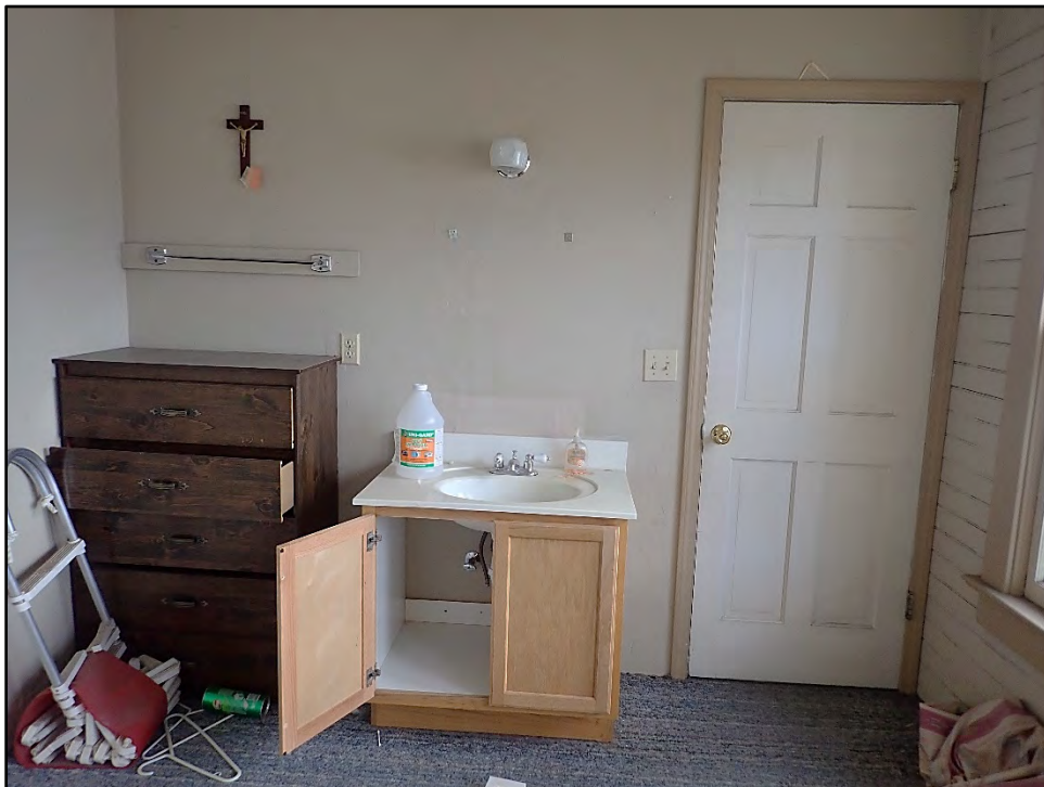
Figure D-480. Detail view of the south wall of the second small bedroom, showing the modern building materials and amenities (including upgraded electrical wiring).
