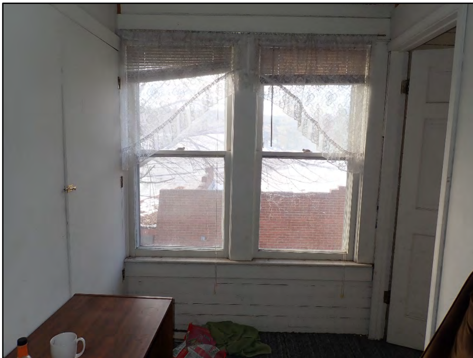
Figure D-486. The original windows of the west wall of the small sitting area on the second floor (on the west side of the residence).
