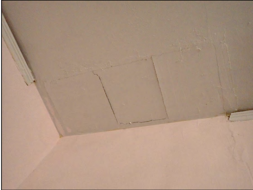
Figure D-435. A view of the ceiling above the corner sink, which reveals portions of the ceiling and walls have been filled in with sheetrock/drywall.
