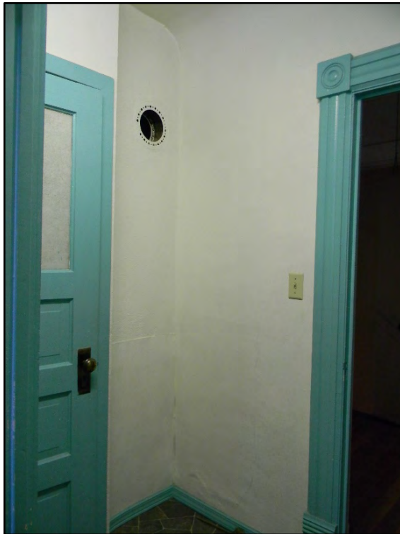
Figure D-514. View of the corner of the large bath (door to the hallway is on the right and small toilet area on the left).
