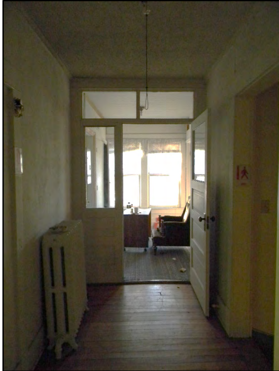
Figure D-511. Looking back down the hallway into the sitting room (the large bath is to the left in this image).
