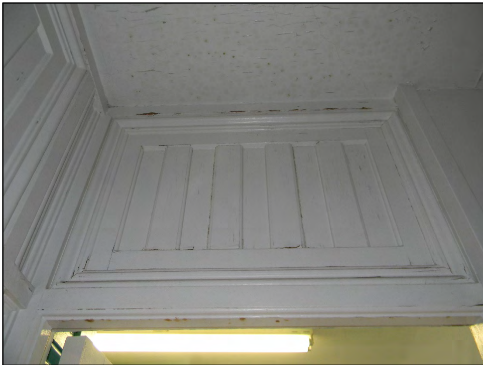
Figure D-526. The original decorative panel above the door to the separate shower.
