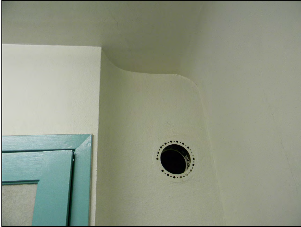
Figure D-515. A detailed view of the ceiling-wall junction showing the curved design of this wall.
