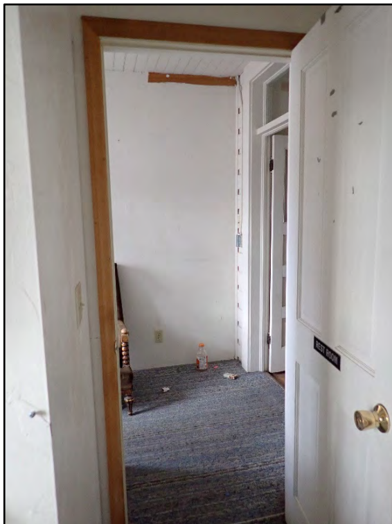
Figure D-502. Looking into the small sitting area through the door to the modern bath.
