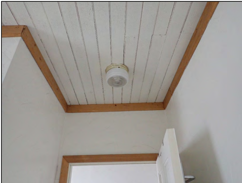
Figure D-500. Detail view of the original wood construction of the ceiling with the modern drywall and trim.
