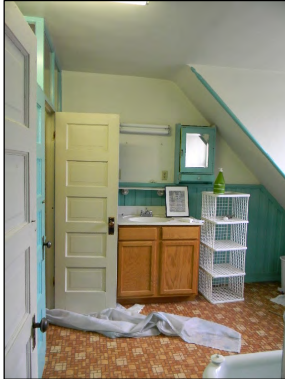
Figure D-527. Overview of the interior of the large bath as seen from the doorway to the separate shower.
