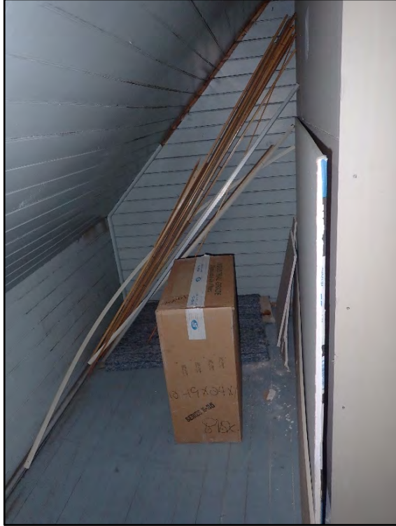
Figure D-497. Interior of the small storage area behind the tub/shower with the original wood batten paneling on the walls and floor.
