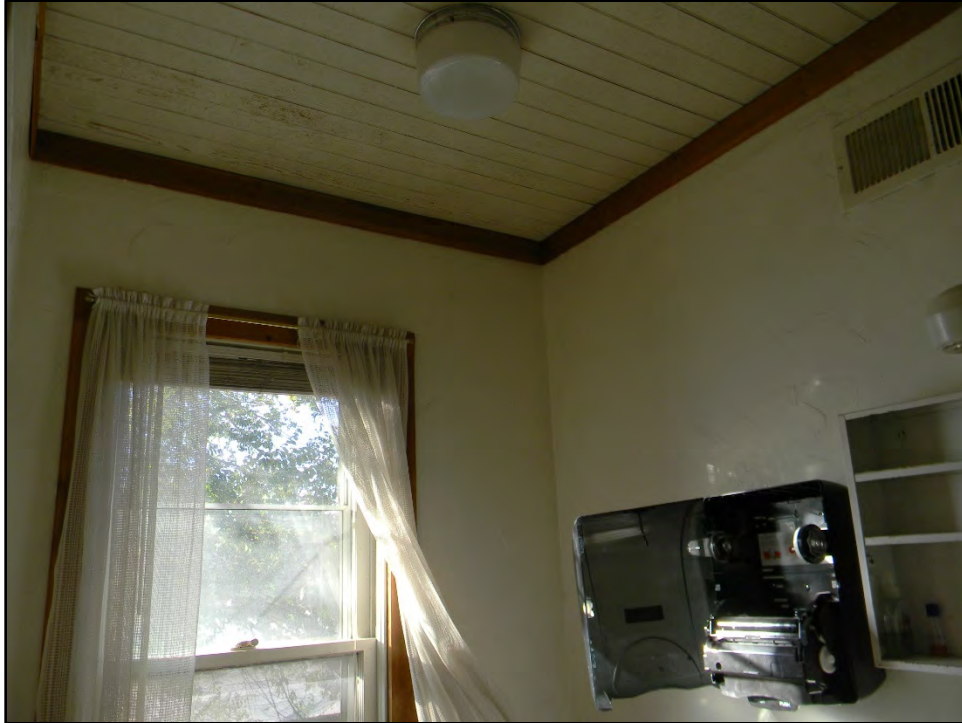
Figure D-493. Detail view of the original ceiling and exterior wall juxtaposed with modern materials incorporated when the modern bath was constructed.
