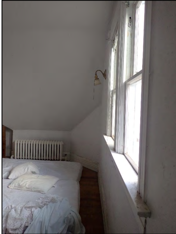
Figure D-559. View along the windows in the gable end.
