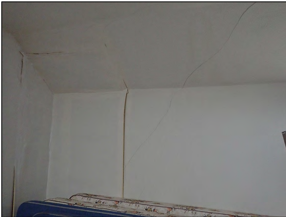
Figure D-606. Cracks and peeled paper affixed to the wall show past repairs and the current condition of this section of the third floor at the northwest corner of the room.
