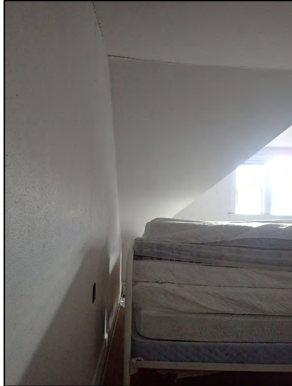
Figure D-565. View of the angled ceiling and wall on the east side of the bedroom (note the cracking and separation at the ceiling juncture).
