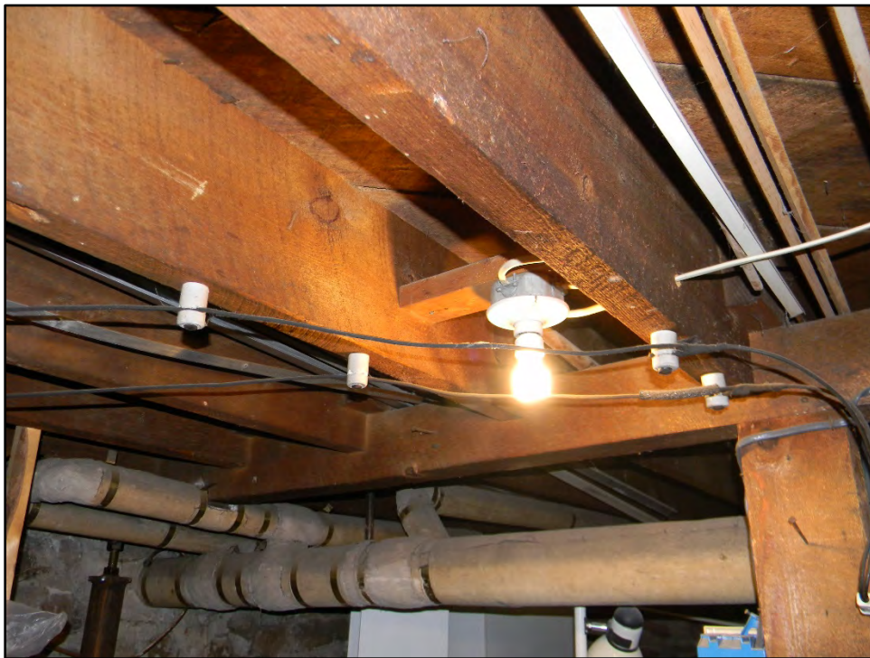
Figure D-624. The floor system of the formal living room, with both historic-era and modern electrical wiring strung underneath.
