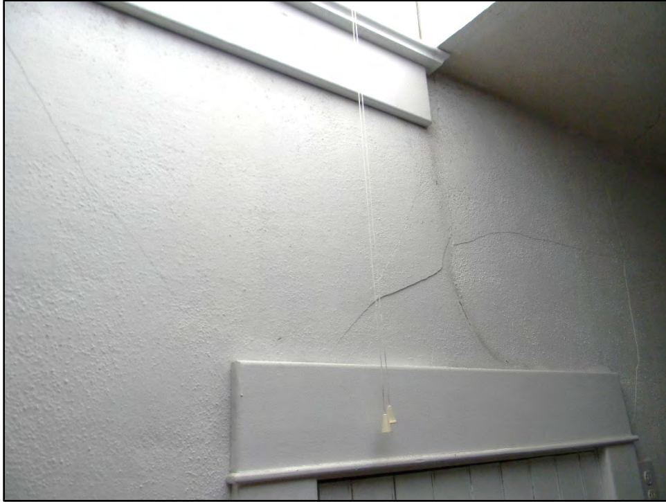
Figure D-581. The sill and apron of the window and the cap trim of the door frame the cracking of the original lath-and-plaster walls.
