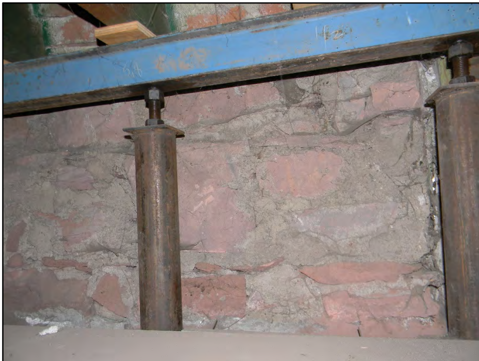
Figure D-630. Shoring jacks have been installed to prevent the collapse of the formal living room, which is structurally compromised.
