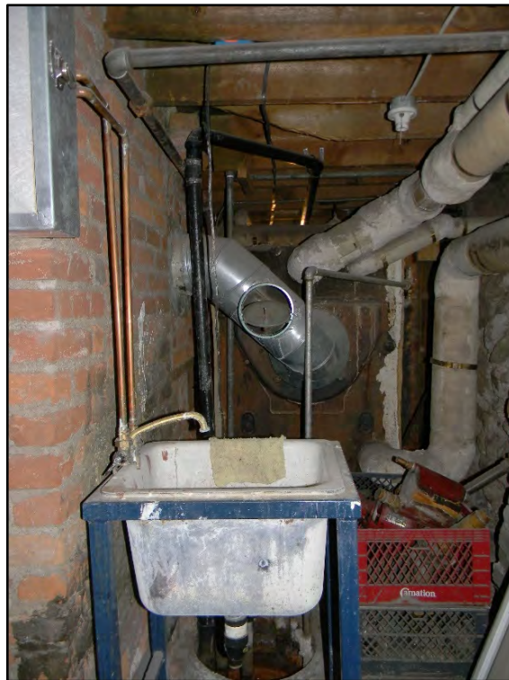
Figure D-622. Modern ducts and utilities weave throughout the basement space.
