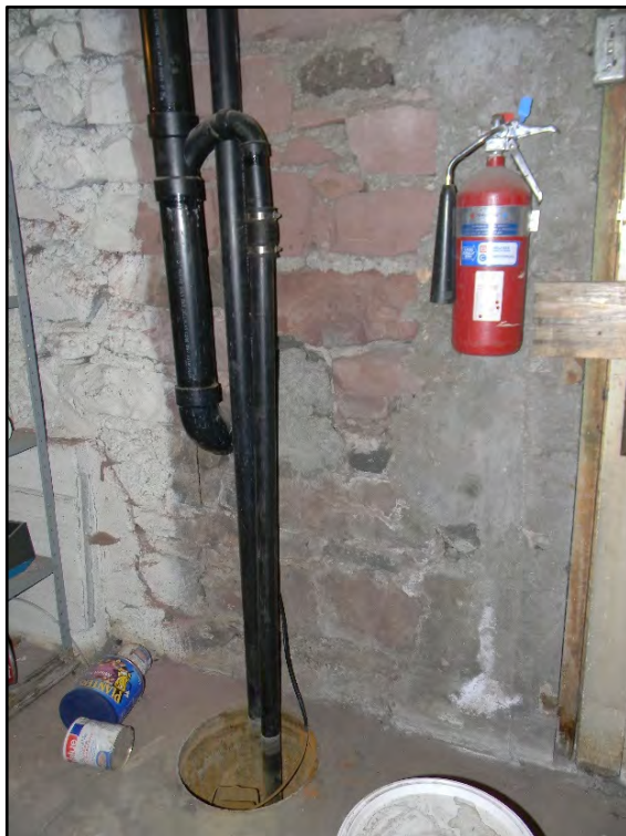
Figure D-638. The sump pump and pit that drains water out of the basement.
