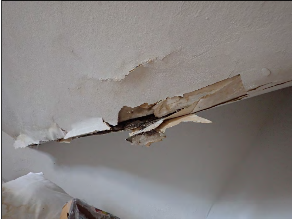
Figure D-563. A close-up view of the rotting wood and ceiling damage.
