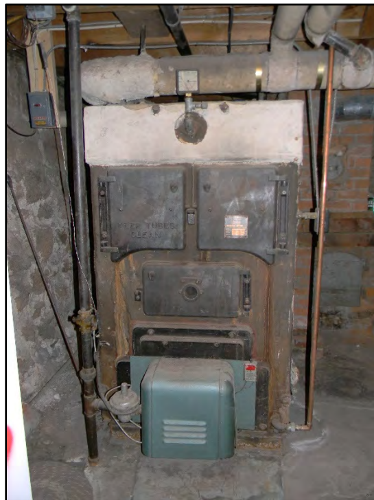
Figure D-618. What is likely the original steam boiler of the residence that feeds to all of the decorative radiators throughout the first and second floors.
