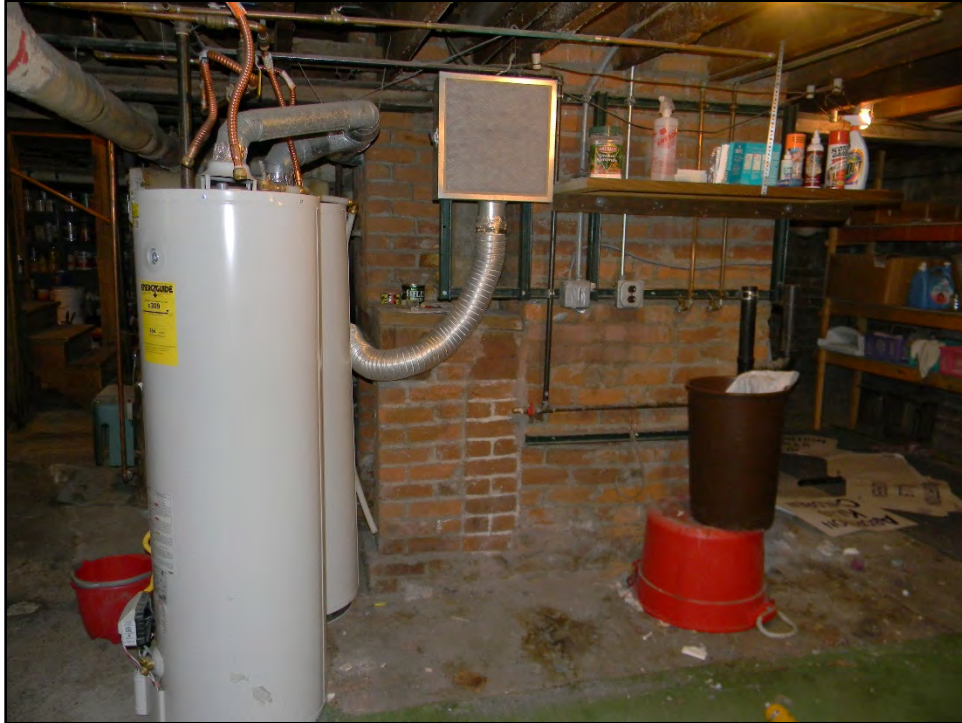
Figure D-619. Modern water heaters installed next to the original brick-and-mortar components of the basement.
