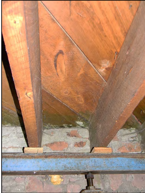
Figure D-631. A detail view of the shoring jacks which now support this part of the first floor under the formal living room.
