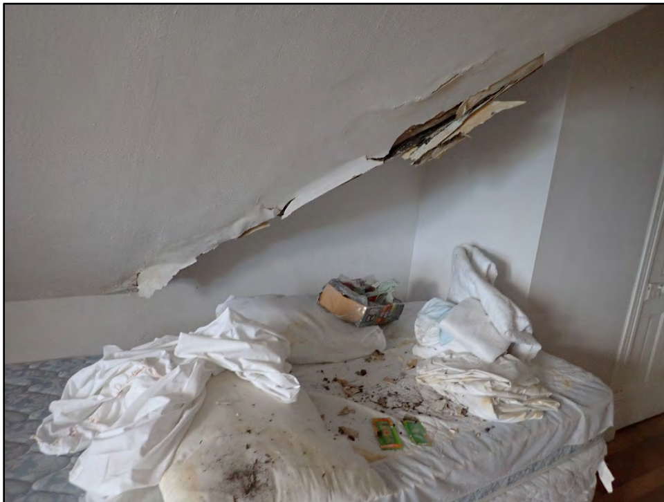
Figure D-562. Detail view of the deterioration and water damage that is present in the fourth bedroom.
