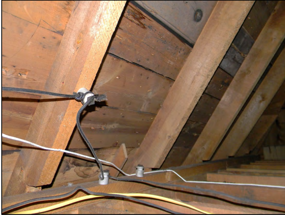
Figure D-587. Another view of the original electrical wiring that is still present in the residence.
