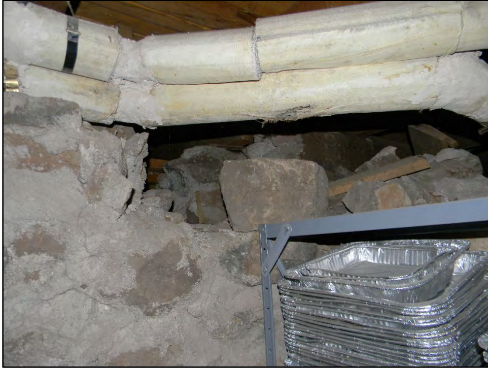
Figure D-663. Portions of the basement walls have collapsed over time.
