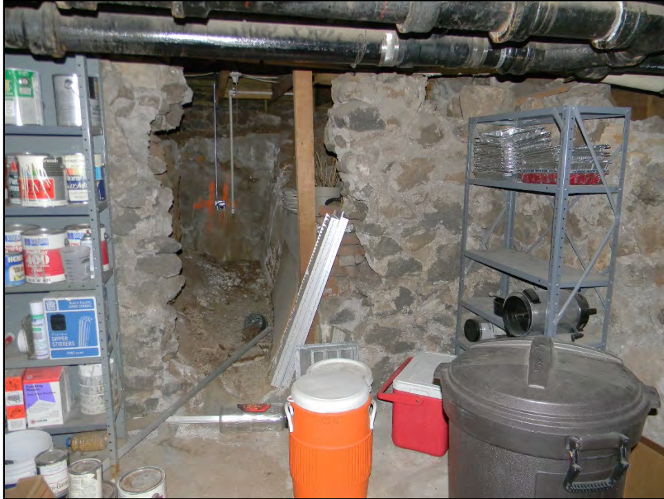
Figure D-659. The northern side of the basement with its original masonry rubble construction (this section likely dates to the earliest period of the residence based on its design and materials).
