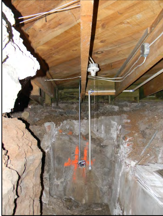
Figure D-661. The floor joists of the first floor atop the stem wall (which is seen at the back).
