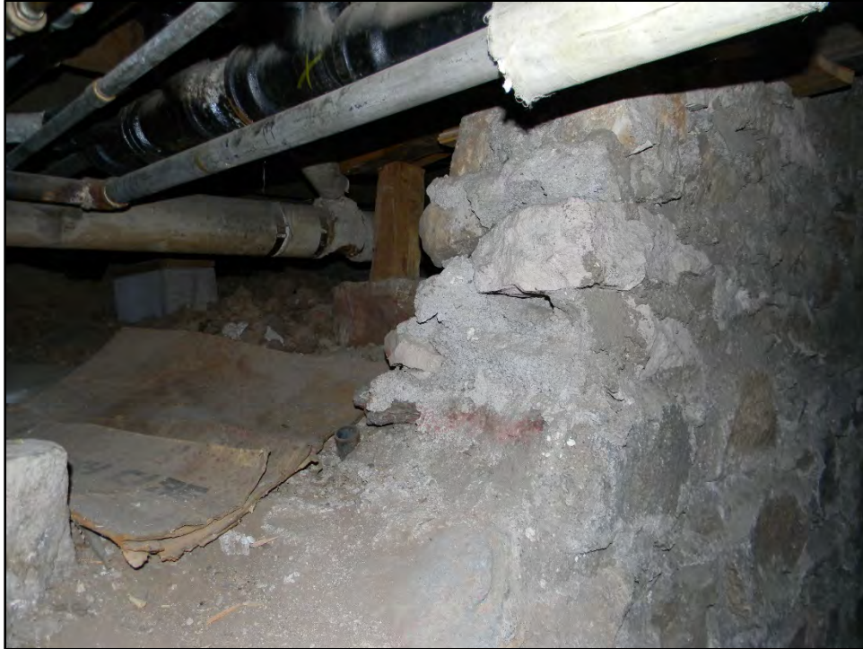
Figure D-665. A detail view of the original masonry construction in the basement dating to the mid-to-late 1880s when the residence was initially built.
