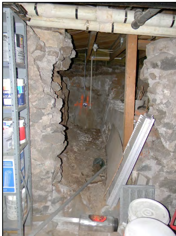
Figure D-660. A detail view of the same crawlspace in the basement.
