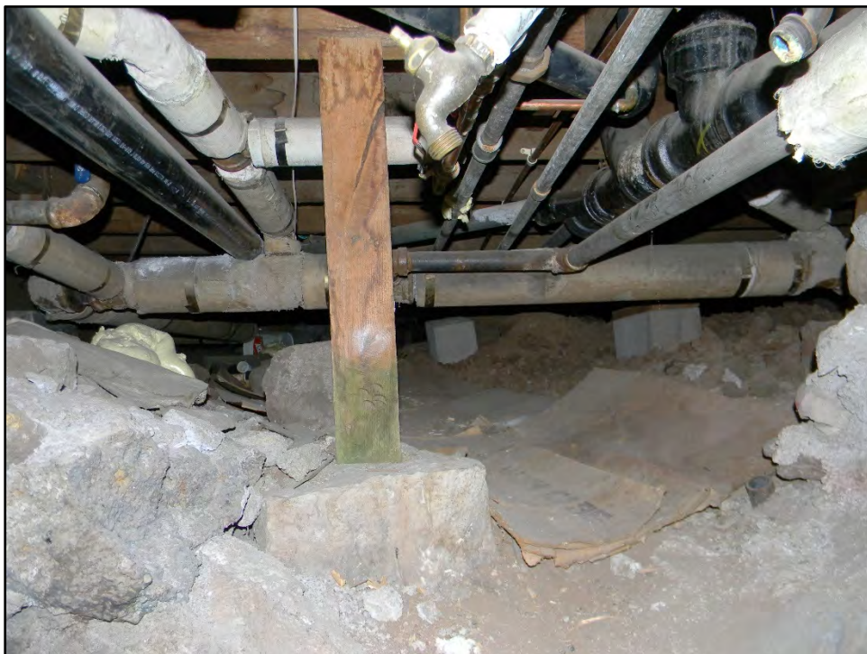
Figure D-664. A detail view of the wood posts and concrete footings that hold up the original extent of the house as built in 1886, which is marked below by this crawlspace which extends back to the stem wall along the North Beaver Street side of the home.
