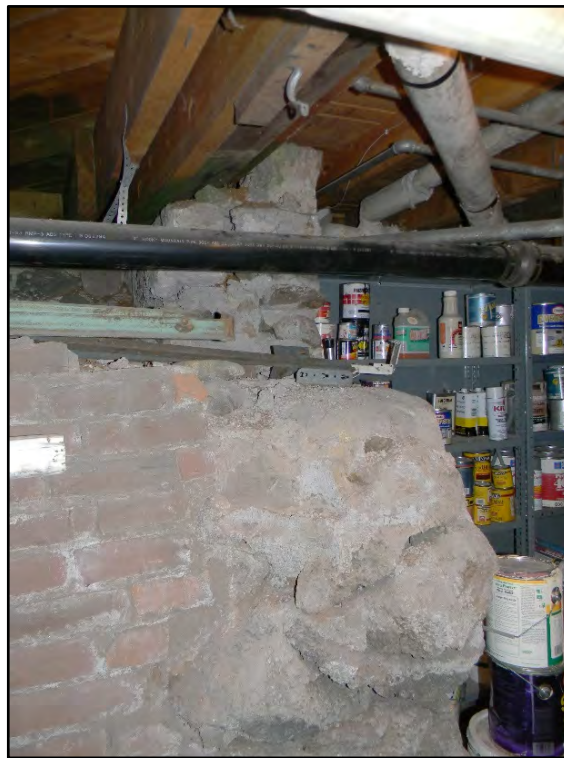
Figure D-658. The north side of the basement has a plethora of brick and rubble masonry retaining walls, the dates and purposes of which remain unknown.
