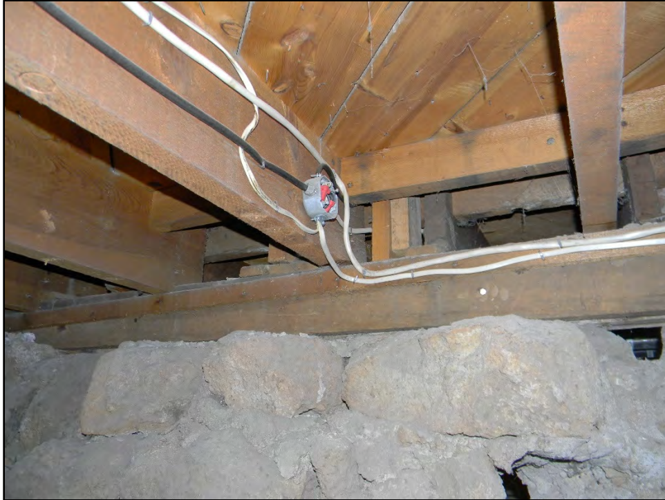
Figure D-657. Detail of the floor system resting atop the basement wall, which is below the main hallway on the first floor.
