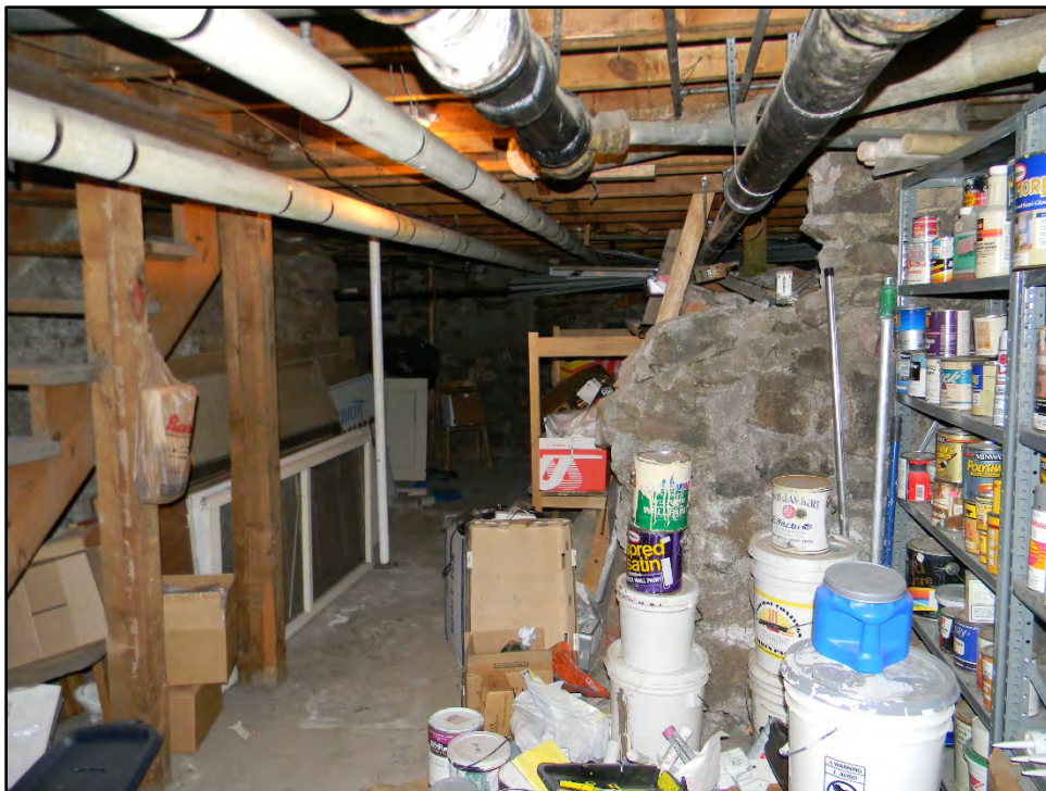
Figure D-666. A glance back toward the well/cistern area of the basement (with the stairs to the first floor at the left).
