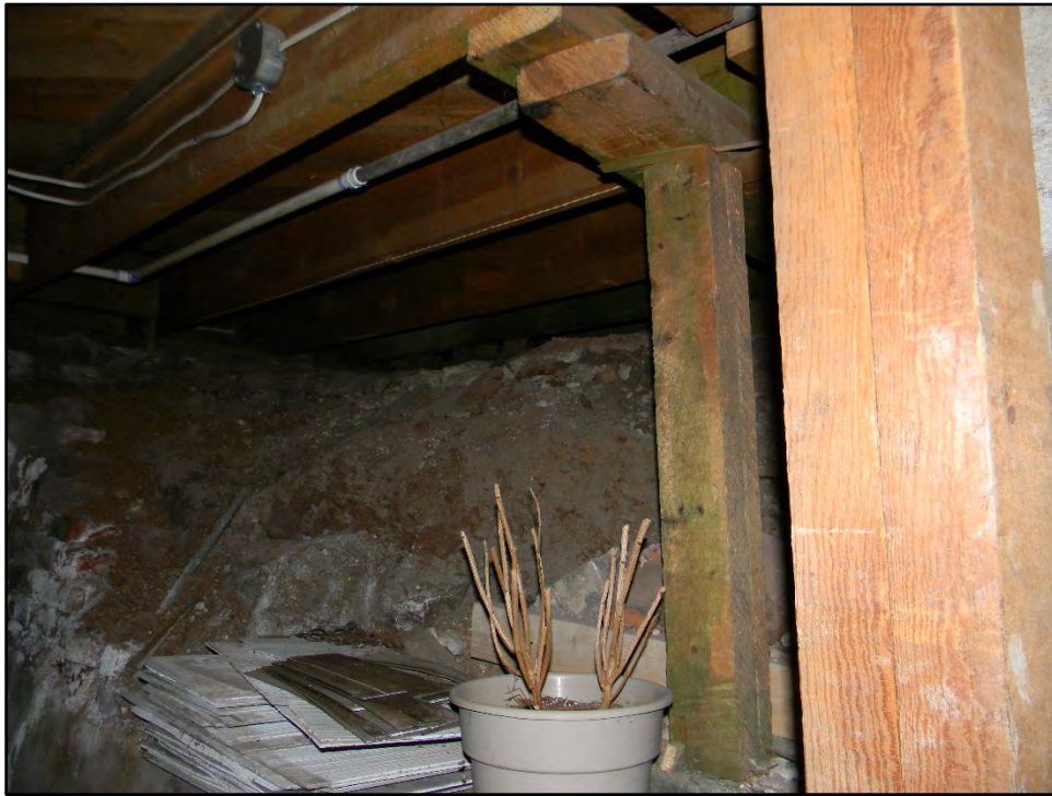
Figure D-662. This image shows the post-and-beam construction of the original extent of the residence (this is below the bedrooms).
