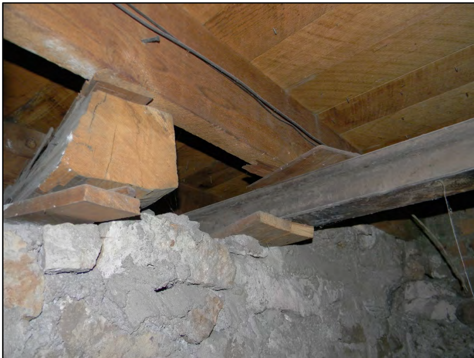
Figure D-668. A close-up view of the steel rail and other materials that still hold up the original 1886 extent of the residence over 130 years later.
