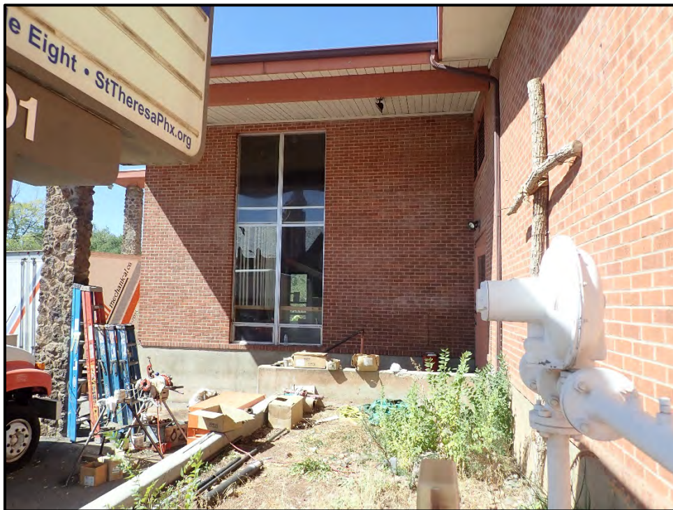
Figure 14. Detail view of one of the window walls of the entrance to the former Catholic school.
