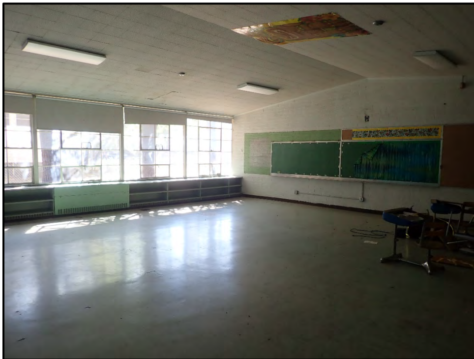
Figure 28. Interior view of one of the classrooms along the east side of the building, showing the walls of windows that lighted each classroom as built in the mid-1950s (note the low-pitched gable ceiling of the original annex).
