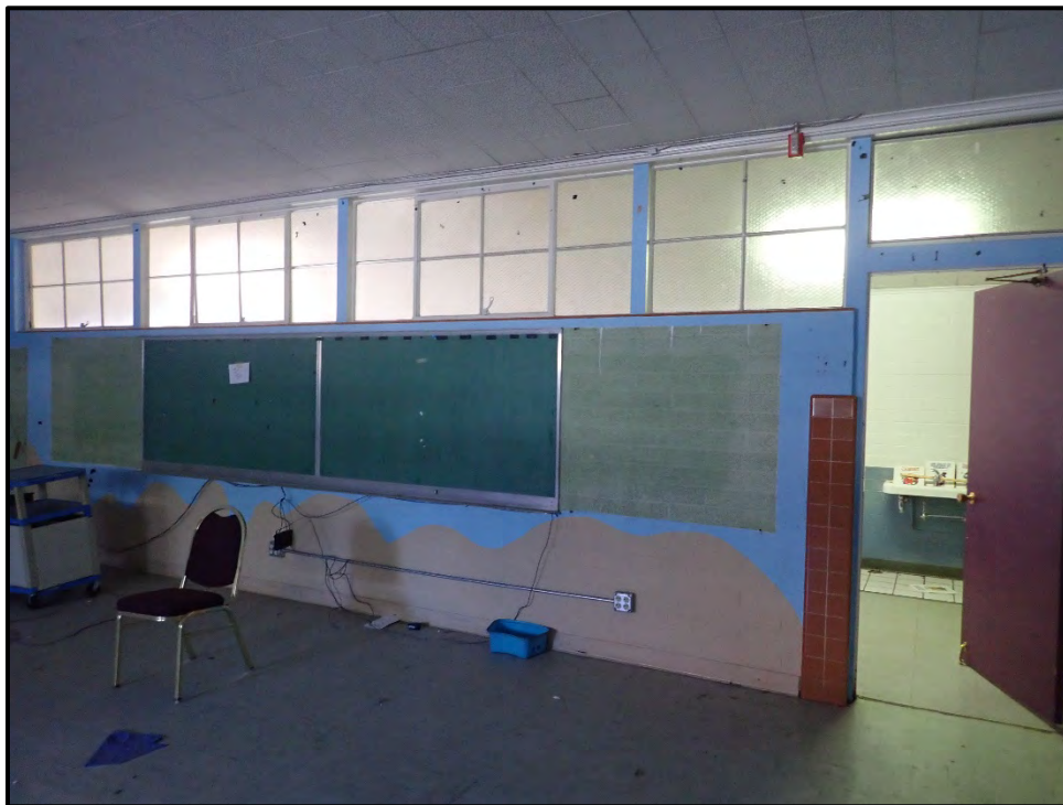
Figure 26. View of the interior of one of the classrooms along the north end of the building, showing the upper windows along the hallway.
