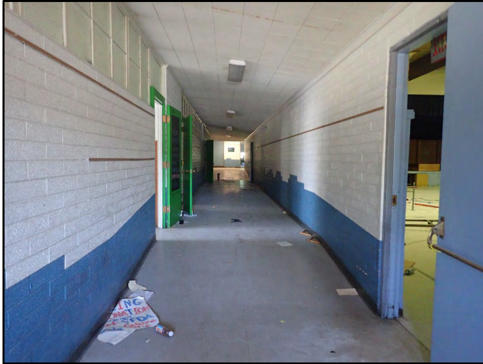
Figure 25. Interior hall along the west side of the school building that was once part of the classroom annex for St. Anthony's Academy.
