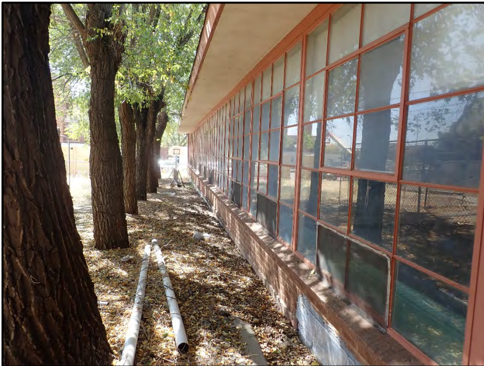
Figure 16. Detail view of the metal windows of the east side of the former Catholic school.
