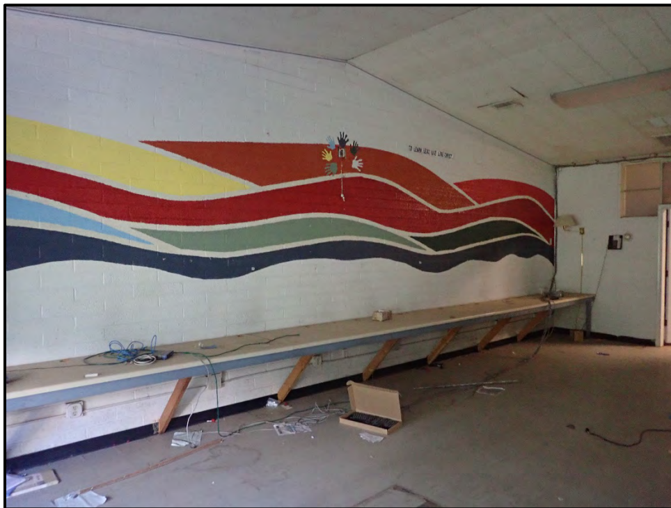
Figure 24. View of the former computer lab located at the north end of the school building.
