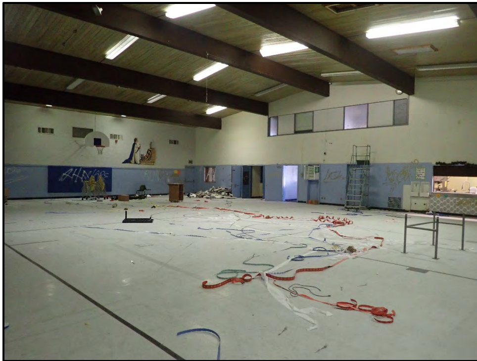
Figure 30. View of the gymnasium (note the upper windows of the music room).
