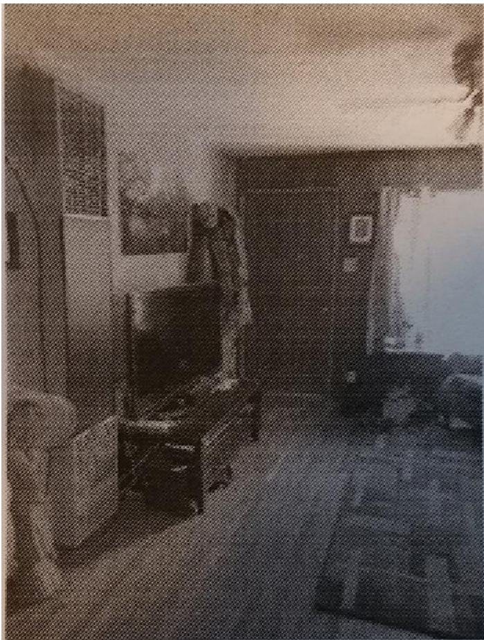
Wall Heater; Foyer; Living Room
