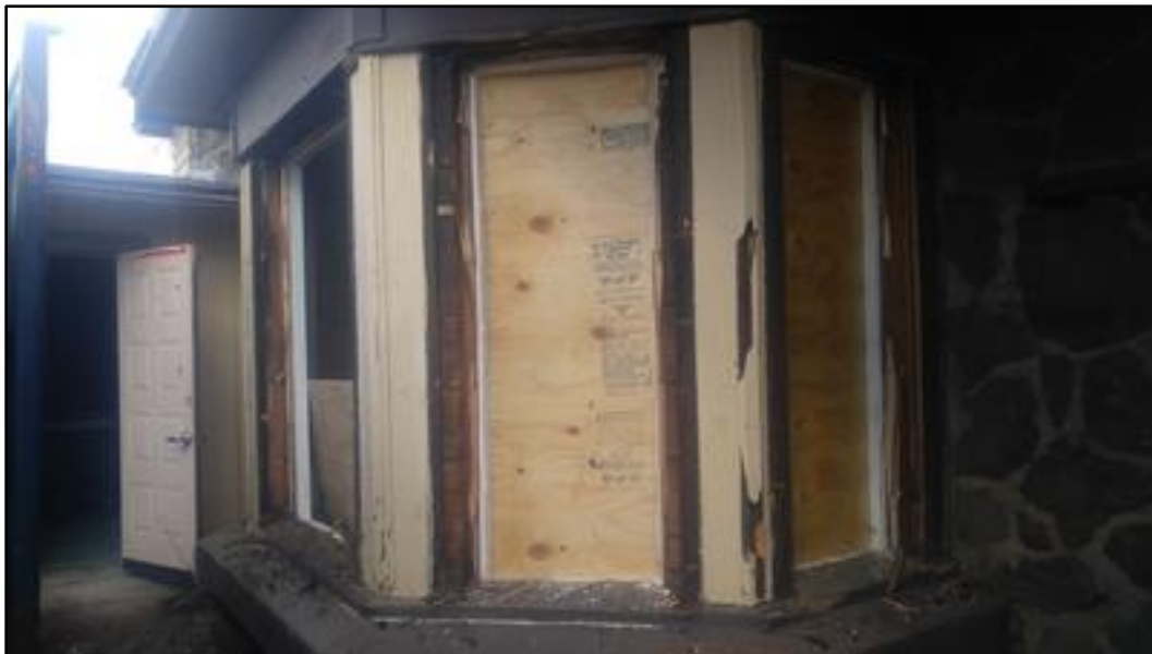
Photograph 33. Entry with cant bay window on the northwest corner of Chapel, facing north.
