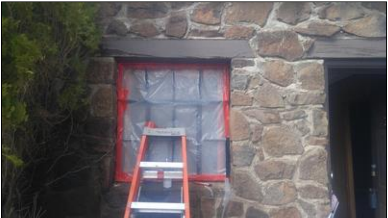
Photograph 35. Window on the Morgue Preparation Room on the east end of the Main Building, facing north.
