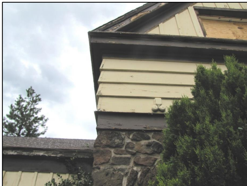
Photograph 20. East second-floor apartment with telephone bell mounted on exterior wall, facing north.
