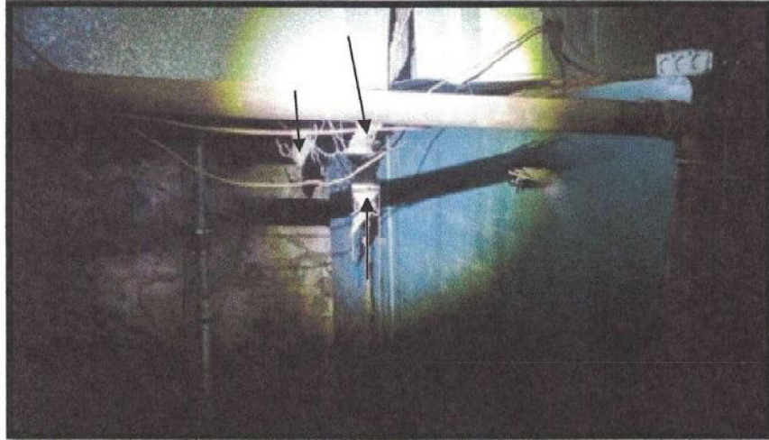
Photo #13: Significantly damaged vibration dampening cloth (VDC) on the boiler ductwork (arrows). The VDC is friable, and assumed to be asbestos containing because it was inaccessible the day of sampling. The concrete boiler room was flooded with 3.5 feet of water from recent heavy rainfall. Viewing northeast inside the boiler room.
