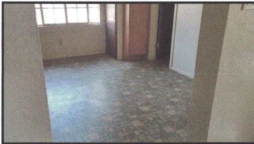
Photo #16: Green linoleum flooring, present in the kitchen and bathroom of the upstairs west apartment, tested positive for asbestos. Viewing down, and to the northeast.
