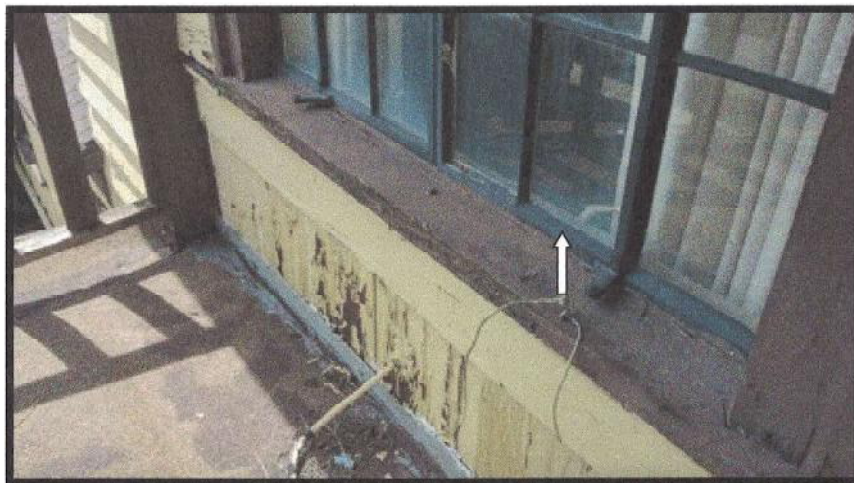
Photo #18: Black painted white window glazing, present on perimeter windows, is reported with a 1-2% chrysotile asbestos content. Viewing down and to the southwest on the upstairs west apartment balcony.
