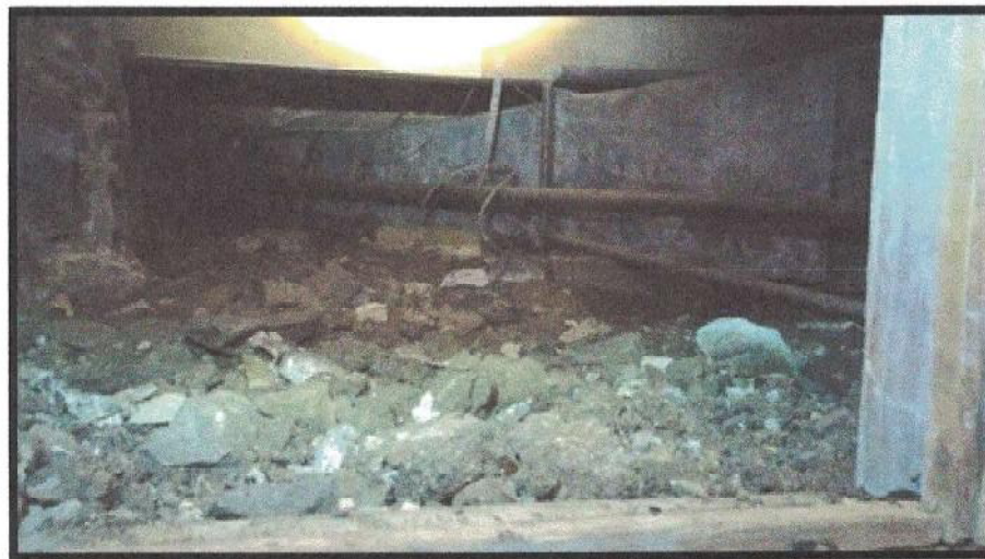
Photo #12: Partial view inside the crawlspace located west of the basement boiler room shows the metal ductwork that leads southwestward toward additions on the west side of the building. Although there is no visible DWI on the metal duct, it appears to be present as debris on the soil. Viewing northwest.
