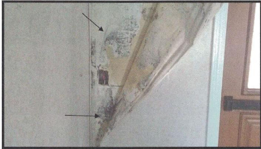
Photo #25: The interior of the chapel contains patterned wallpaper with well-developed mold contamination at a location of water-damage (arrows). The mold appears to be the result of a roof leak that drained down the interior of the wall system. Viewing northwest.
