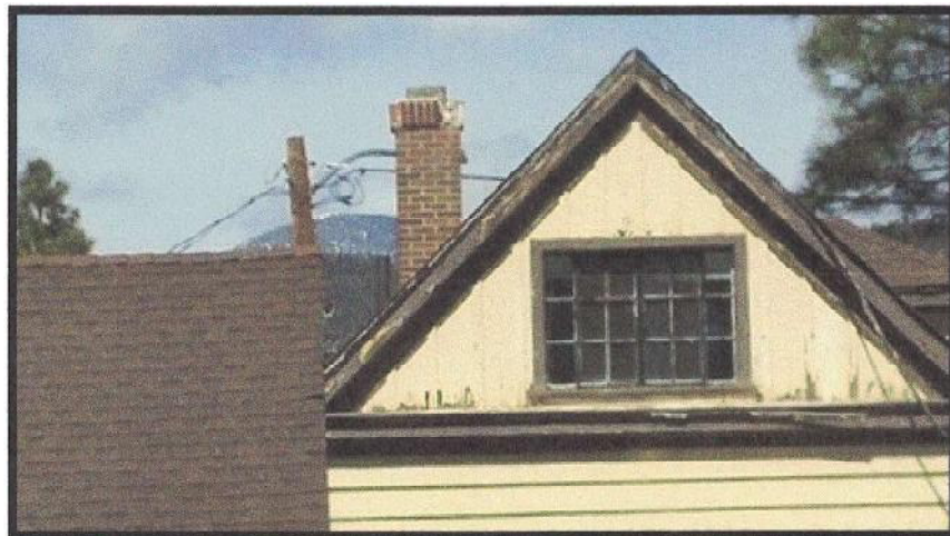
Photo #14: Roof dormer on upstairs east apartment accessed by entering the office. Viewing northwest.
