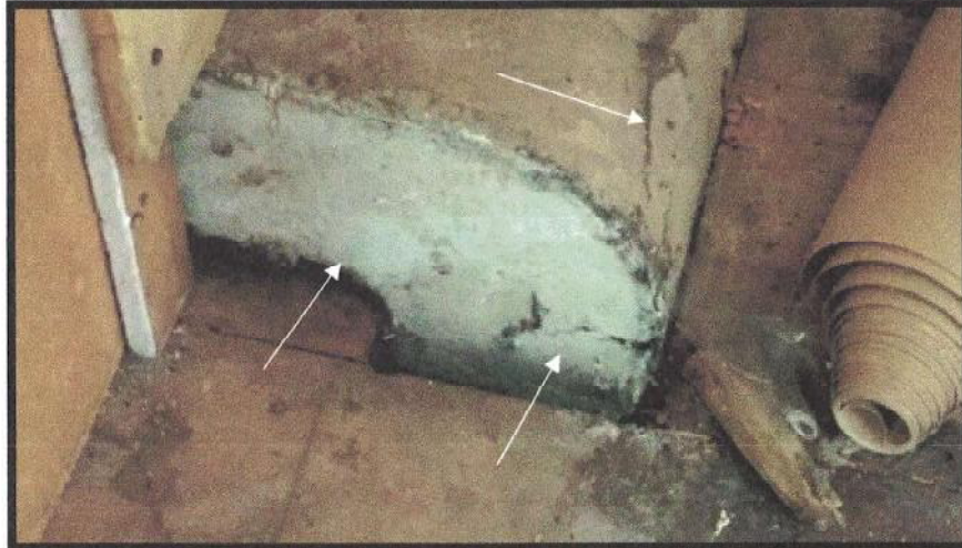
Photo #11: Inside the preparation room is a closet with a portion of a metal duct that connects to a boiler in the basement. The friable (easily crumbled with hand pressure, when dry), white duct wrap insulation is significantly damaged, and suggestive of incomplete removal. The duct wrap insulation (DWI) is reported with a 20-30% chrysotile asbestos content. Viewing down, and to the southwest.
