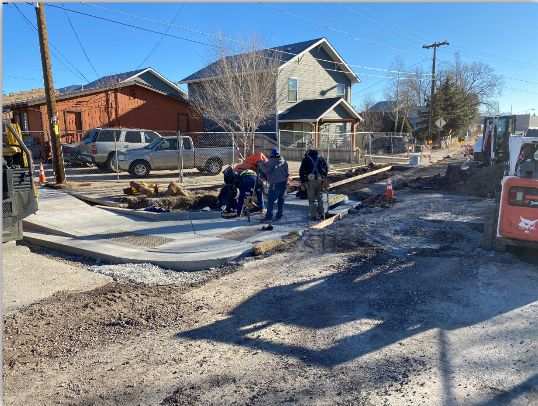
Kingman/Clay intersection looking east at final sections of concrete being prepared for replacement.
