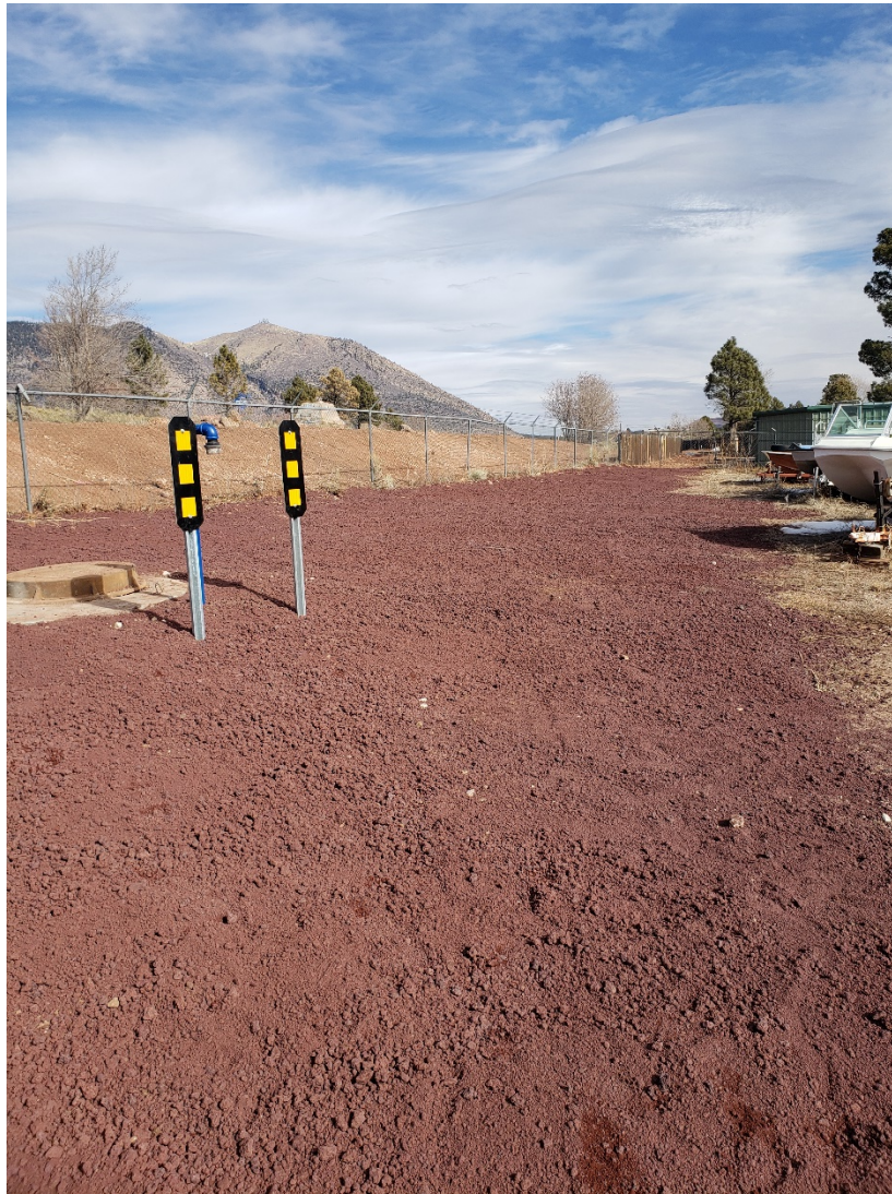
Huntington Waterline Replacement, looking east at final grading and stabilization of the easement
