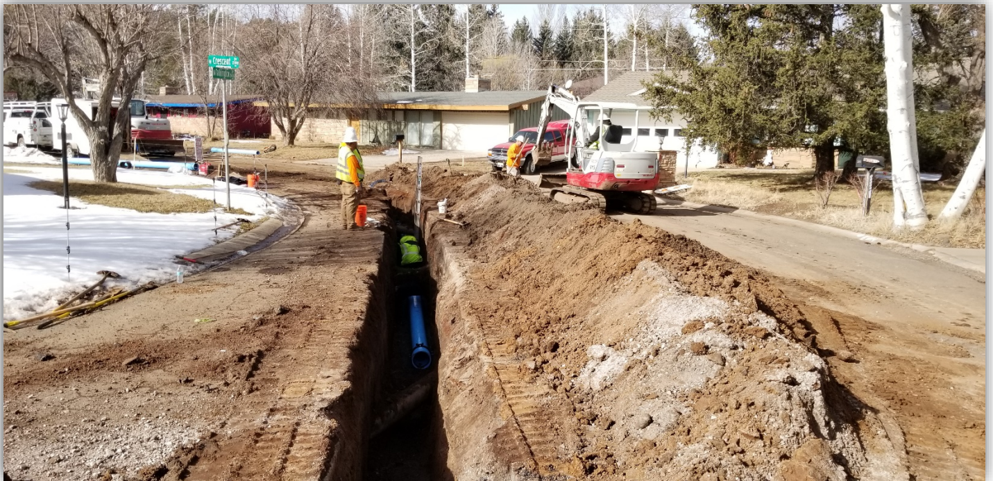
Crescent Dr. at Talkington corner, looking northwest at new water main construction.
