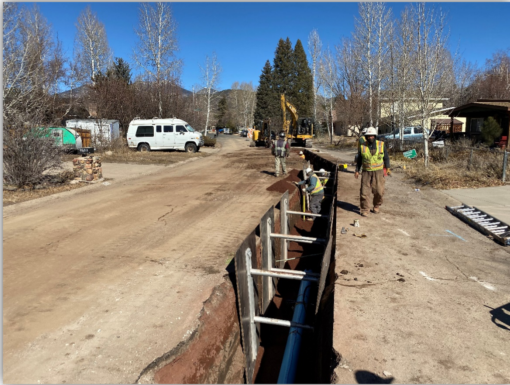
Navajo Dr. south of Anderson Dr., looking north at the water main and service installations.
