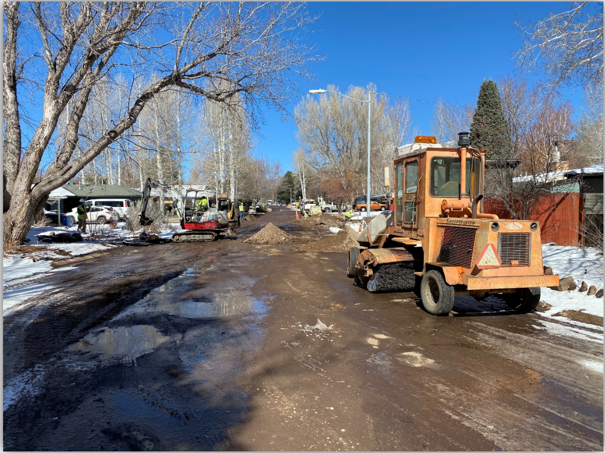
Navajo Dr. at Elizabeth Dr., looking north at final water service installations.
