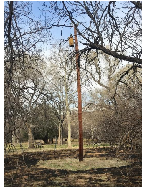
Example of Defensible Space Around Poles
