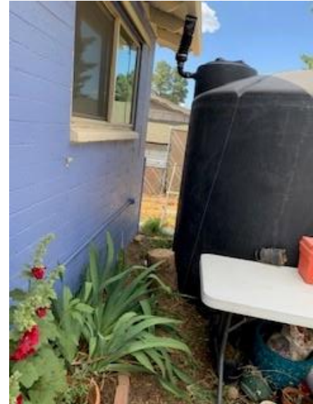
Rain catchment barrel installed at the Greenlaw Garden Hub to reduce water use by supplementing irrigation with rain water.
