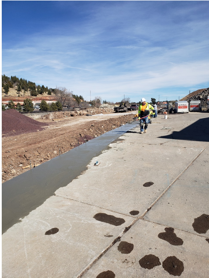
Huntington Waterline Replacement, crews working to finish concrete work at U-Haul related to the waterline replacement
