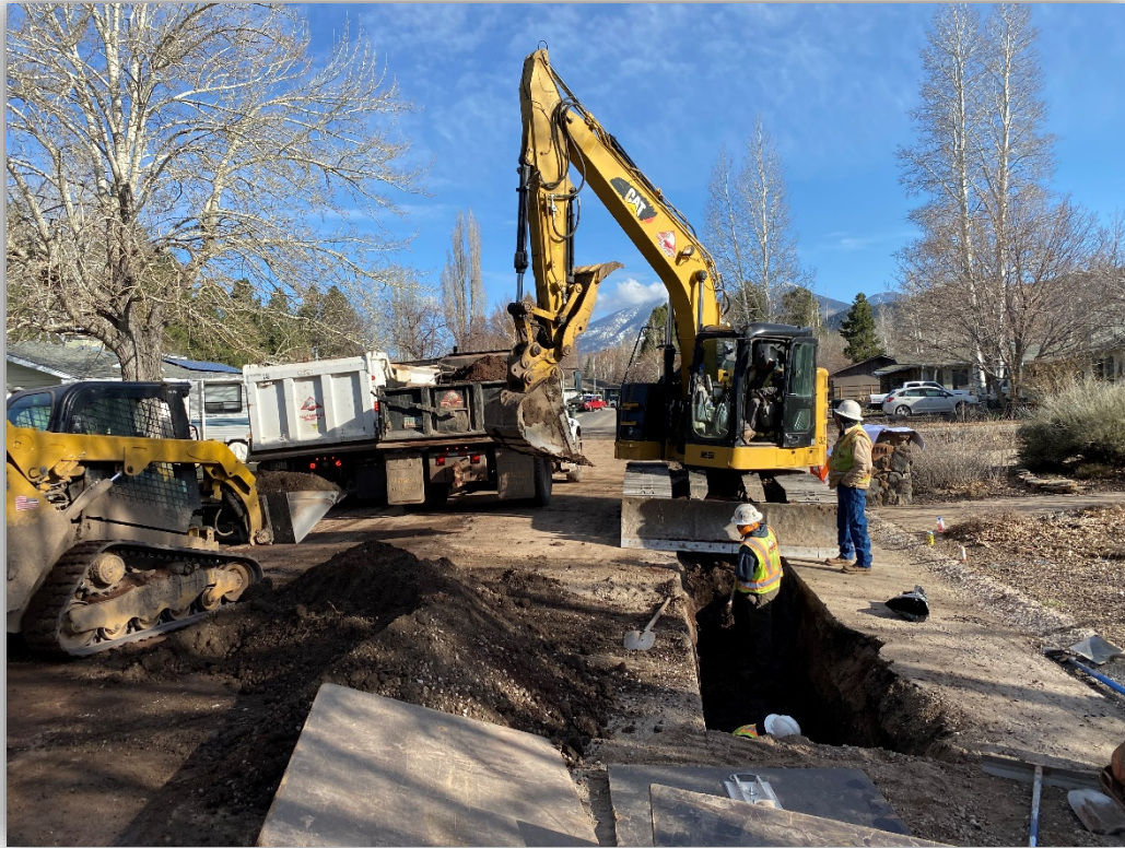
Navajo Dr. north of Anderson Dr., looking north at the water main and service installations.
