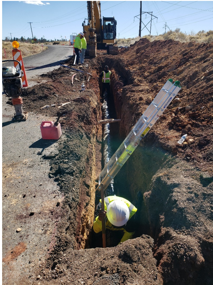
El Paso Flagstaff Rd., looking south at the start of the installation of the 8” ductile iron waterline
