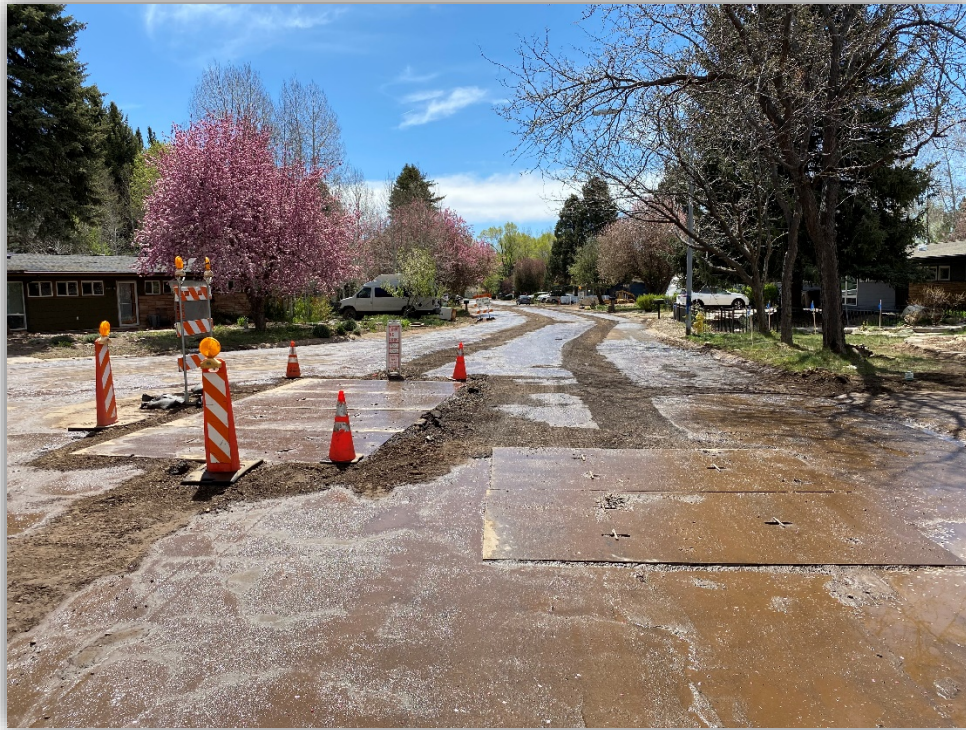
Talkington/Louise intersection, looking south at completed sewer main installations and beginning of water main installations.
