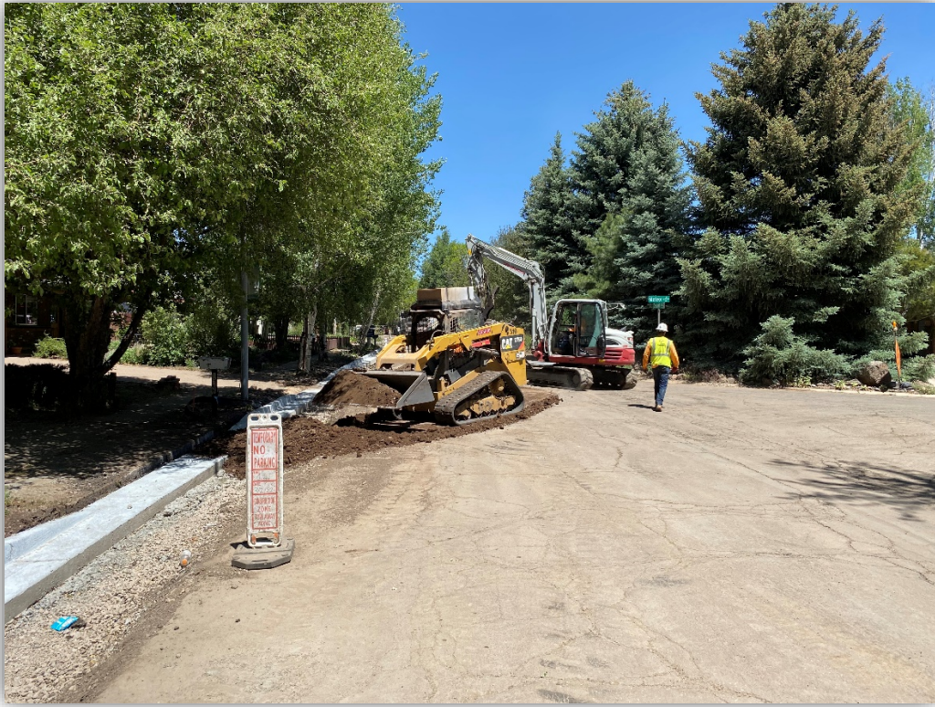
Crescent/Meteor north intersection, looking north at concrete curb installations and temporary driveway ramp installations.
