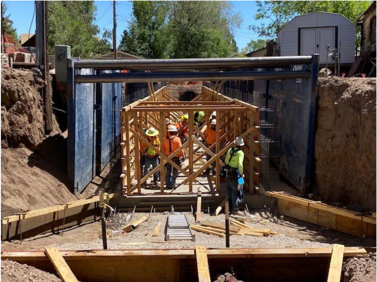
Walls and top of structure being formed. Floor is installed. Looking south.
