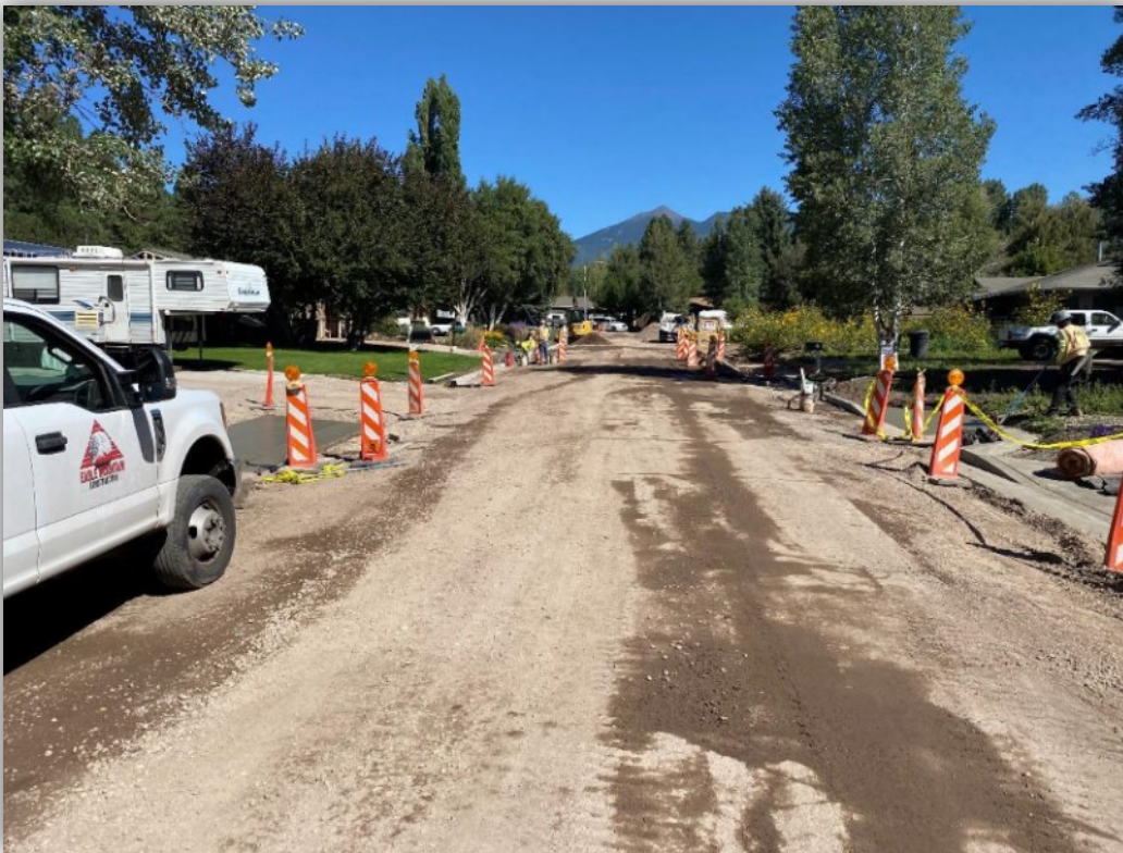
N Navajo Dr. at Murray Rd., looking north at completed curb installations up to Murray.
