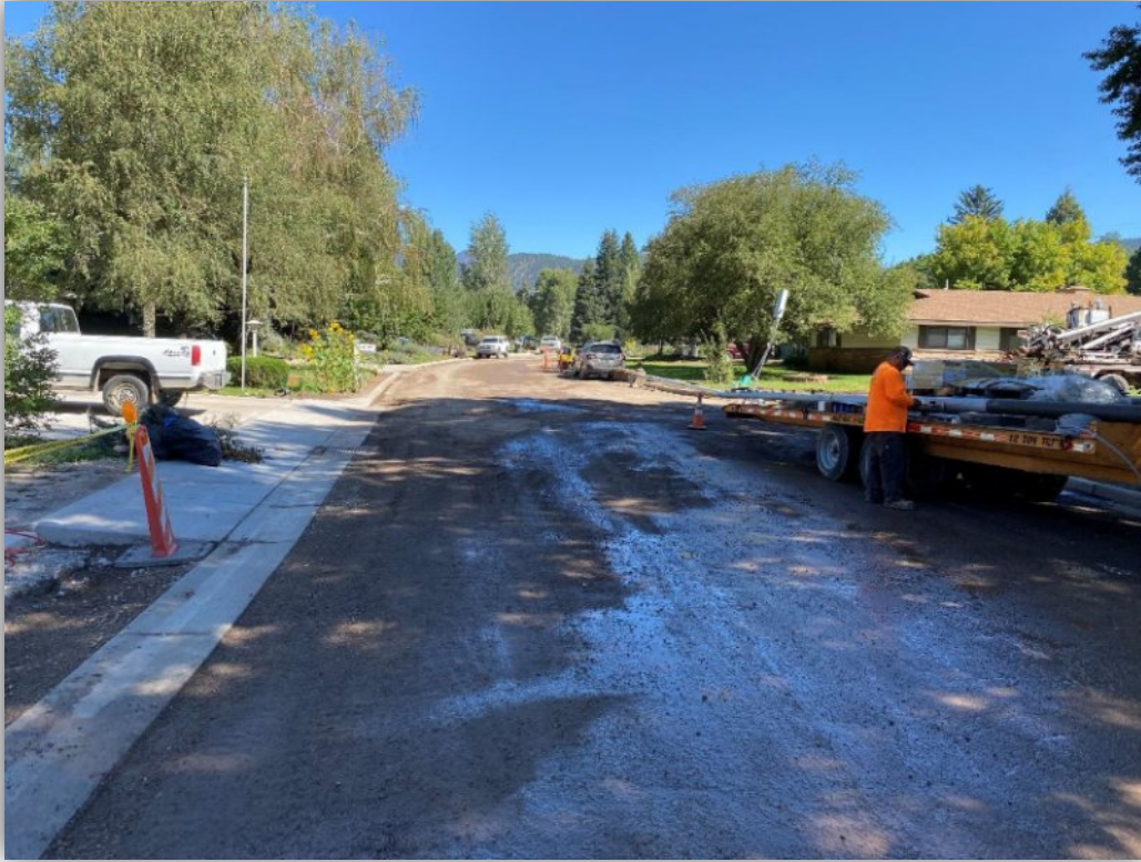
N Navajo Dr. at Whiting Rd., looking north at streetlight installations.
