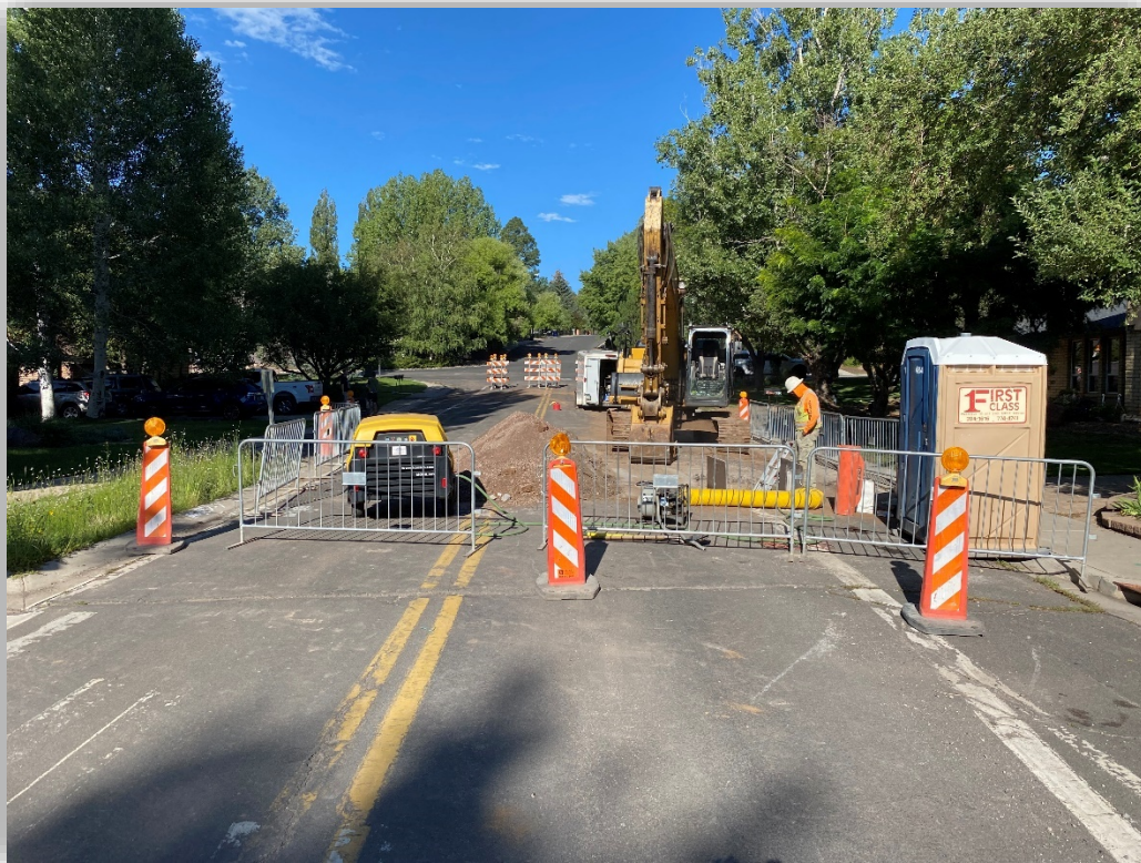
Navajo Dr. at Whiting Rd., looking north at the concrete curb and gutter installations
