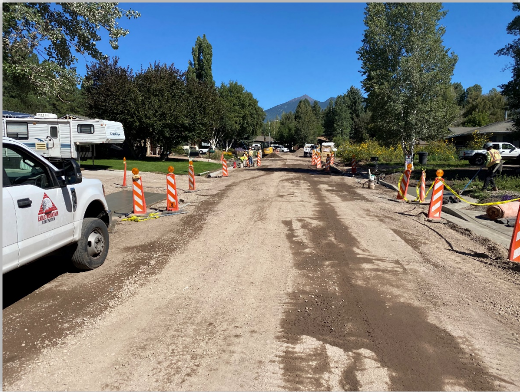
N Navajo Dr. at Murray Rd., looking north at completed curb installations up to Murray.
