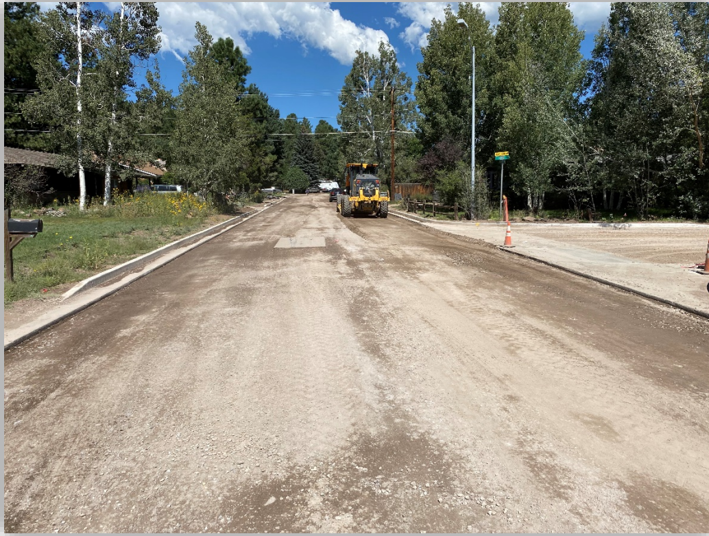
Crescent/Azure intersection, looking north at final roadway grading prior to roadway paving on September 7-9
