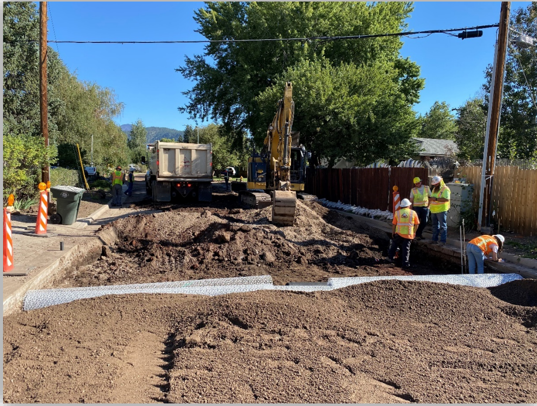
N Navajo Dr. at Murray Rd., looking at water and sewer installations.
