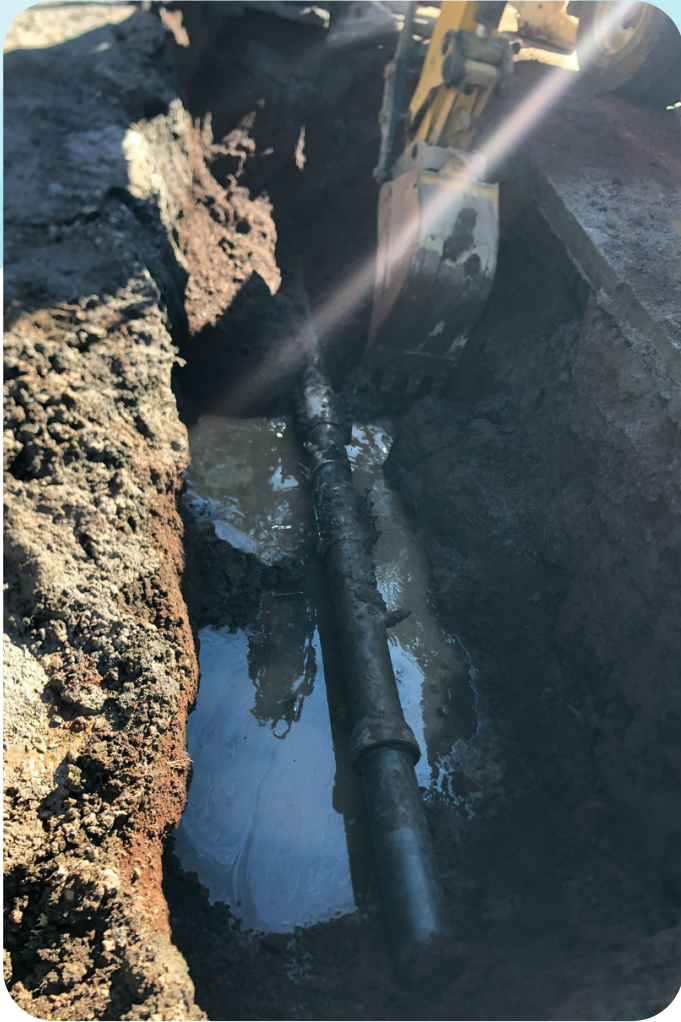
Emergency crews excavated and repaired several breaks along a 1962 6" cast iron main on Silver Spruce Ave.
