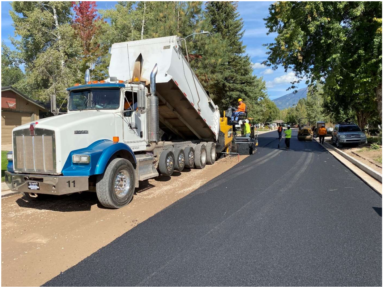
Navajo Dr. north of Anderson Rd., looking north at roadway asphalt paving.
